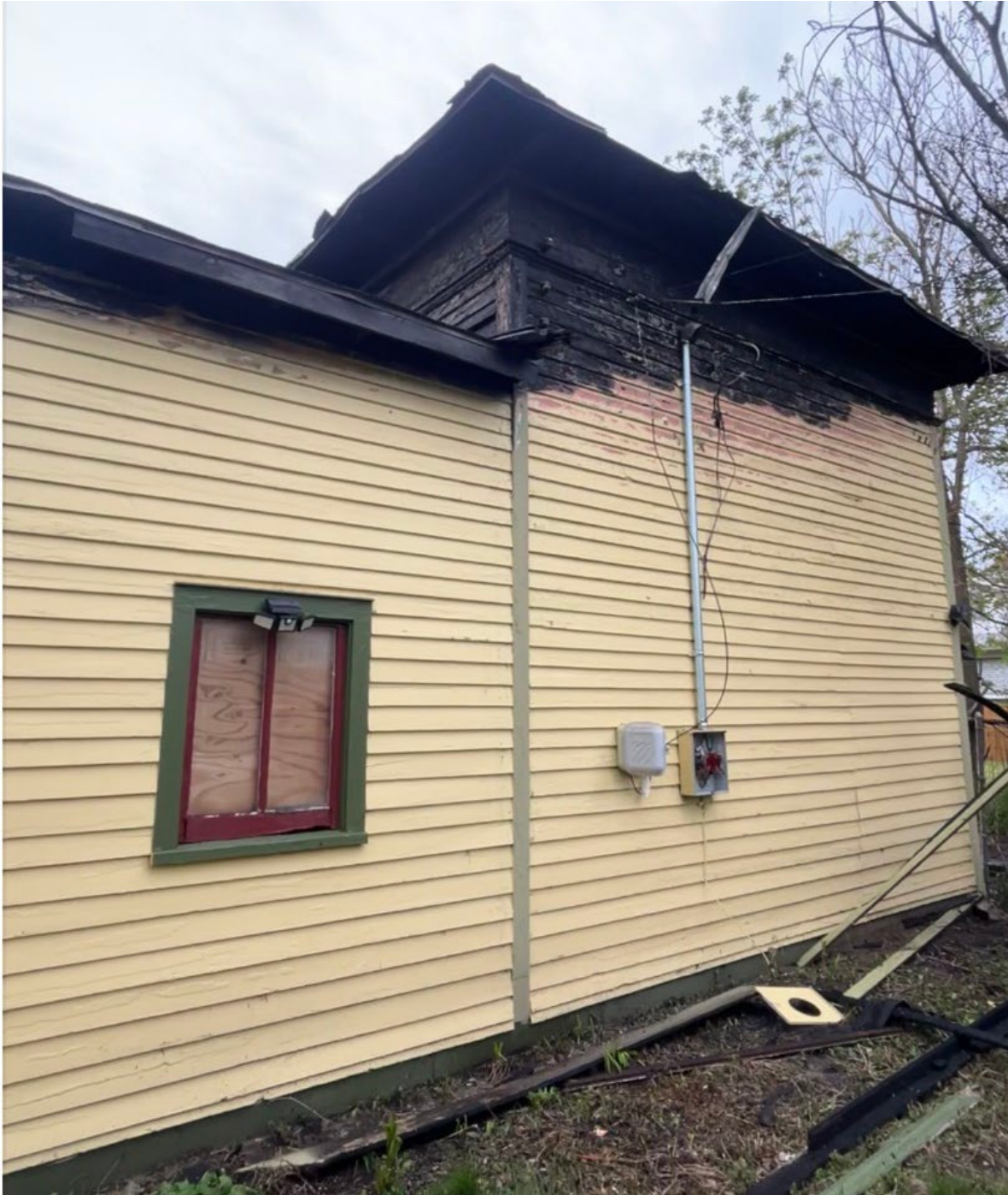
View of rear elevation after the fire, but before demolition.
