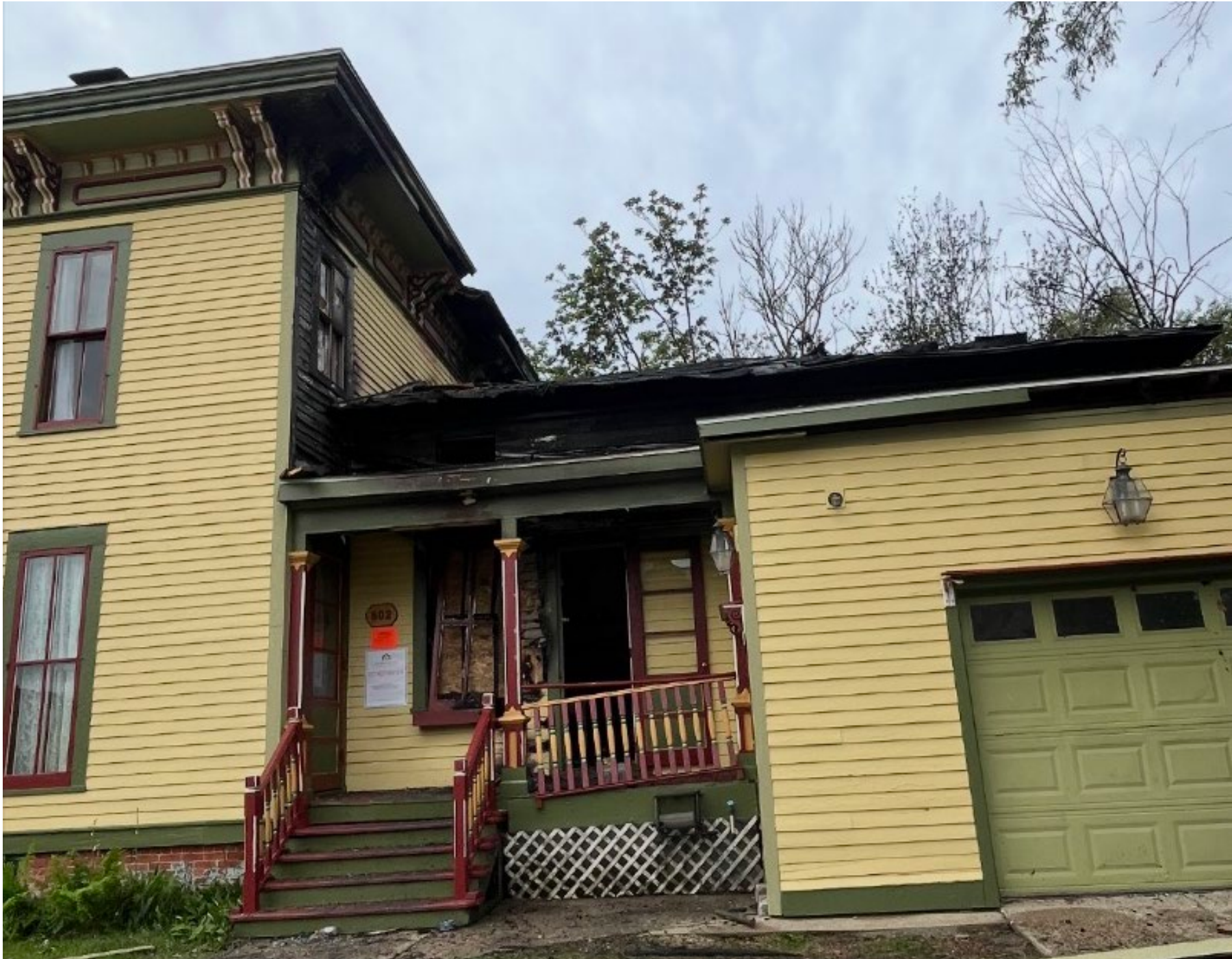
View of rear addition from 6 th Street after the fire, but prior to demolition of roof and garage.
