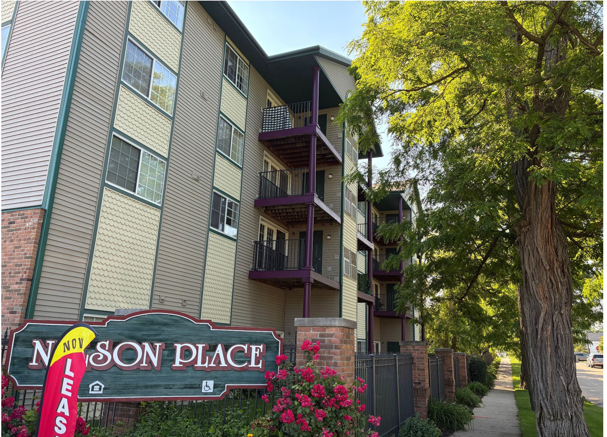
View of two sets of Stack 1 balconies from the corner of W. Muskegon Avenue and 5 th Street, looking southeast.
