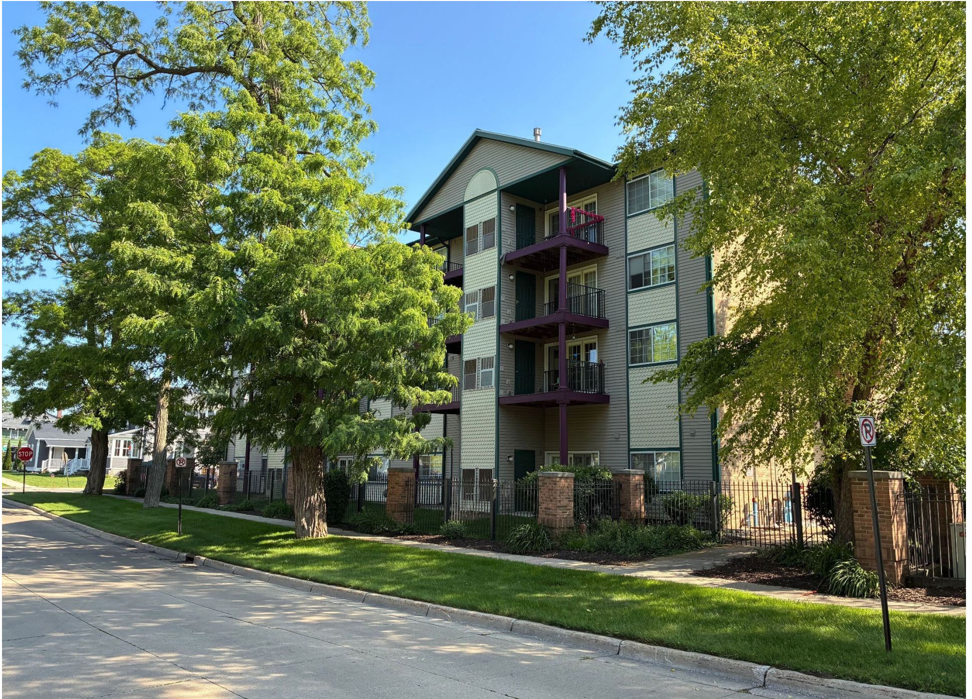
View of Stack 1 balconies from 5 th Street, looking north; railings have been temporarily relocated to prohibit use of the unstable balconies.
