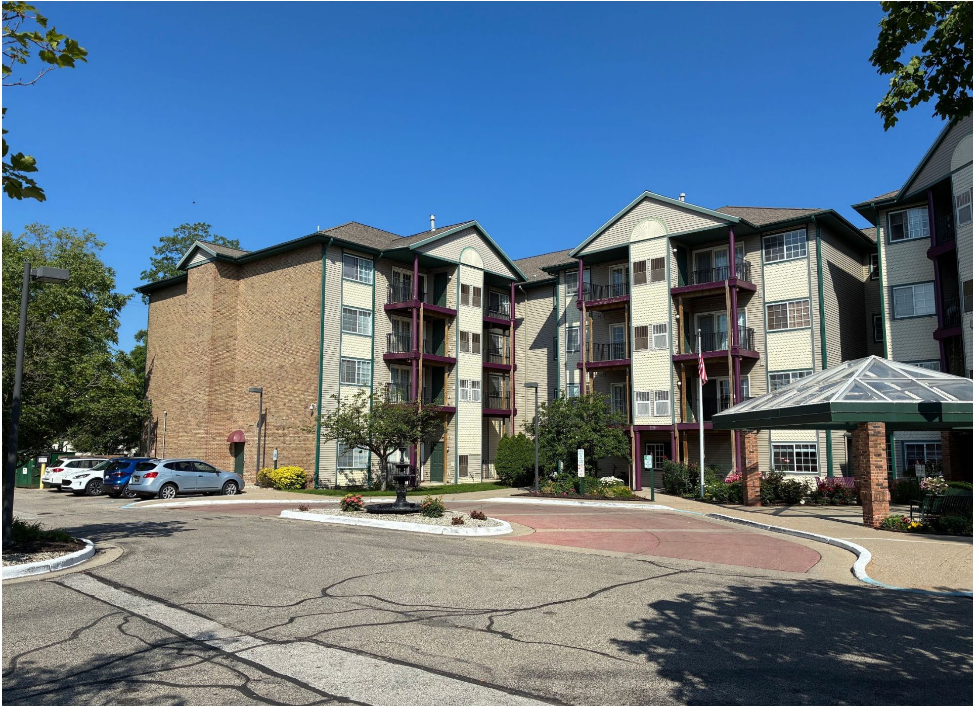
View of Stack 1 and 2 balconies from parking lot, looking west; temporary columns used for reinforcement are visible.
