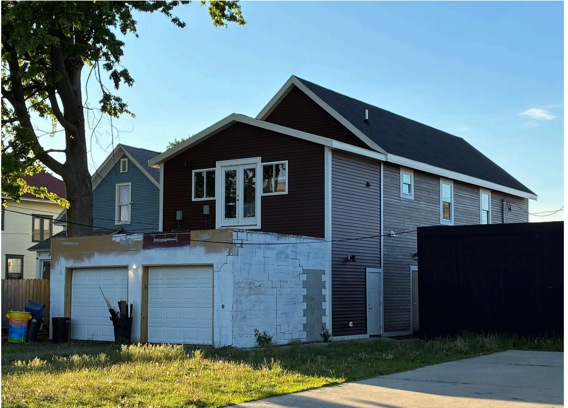
View of rear deck from rear alley, looking east; French doors (that replaced former slider door) visible.
