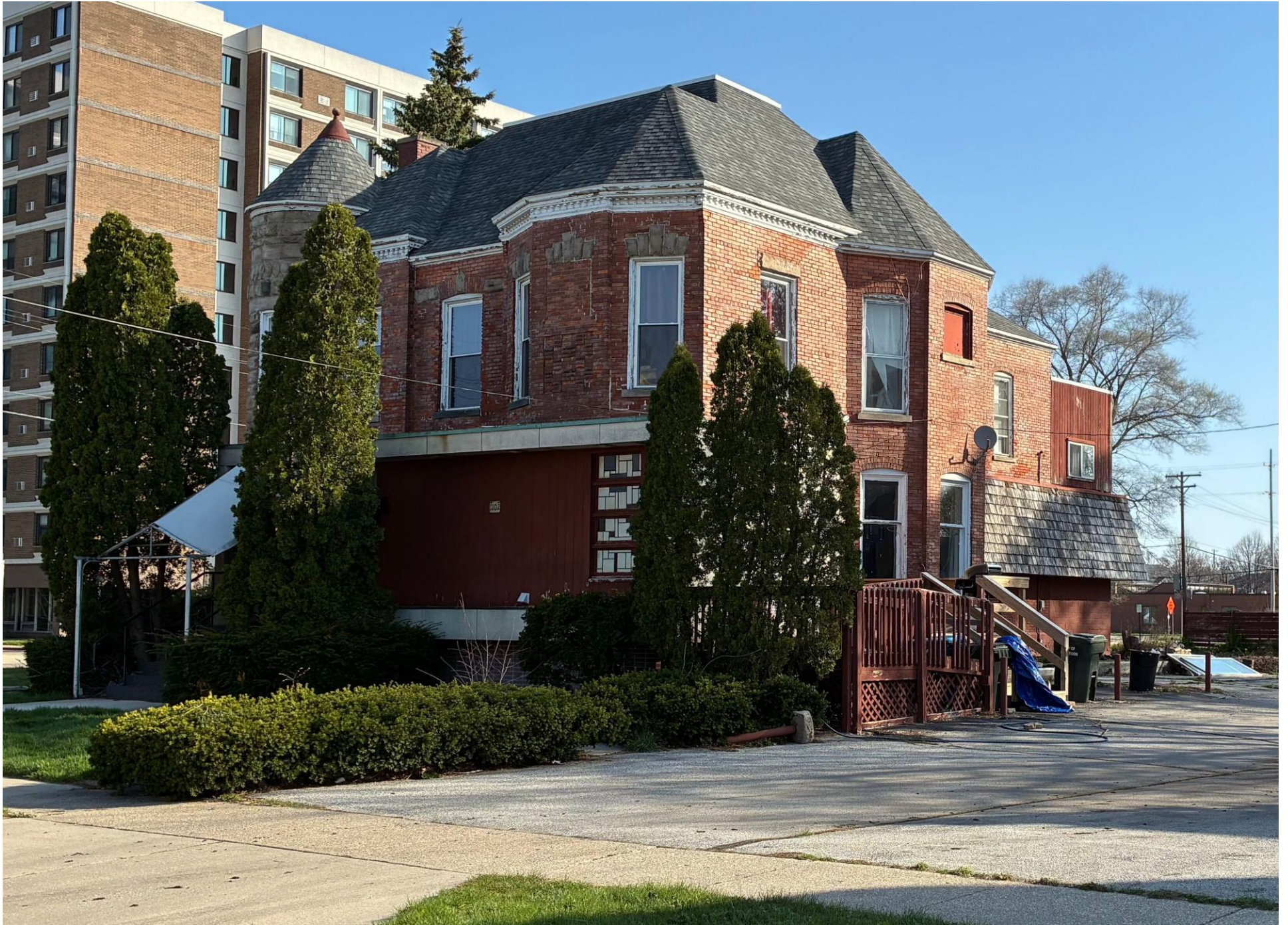
West (front) and south (side) elevations from Terrace Street, looking northeast; deck and former ramp visible at right.
