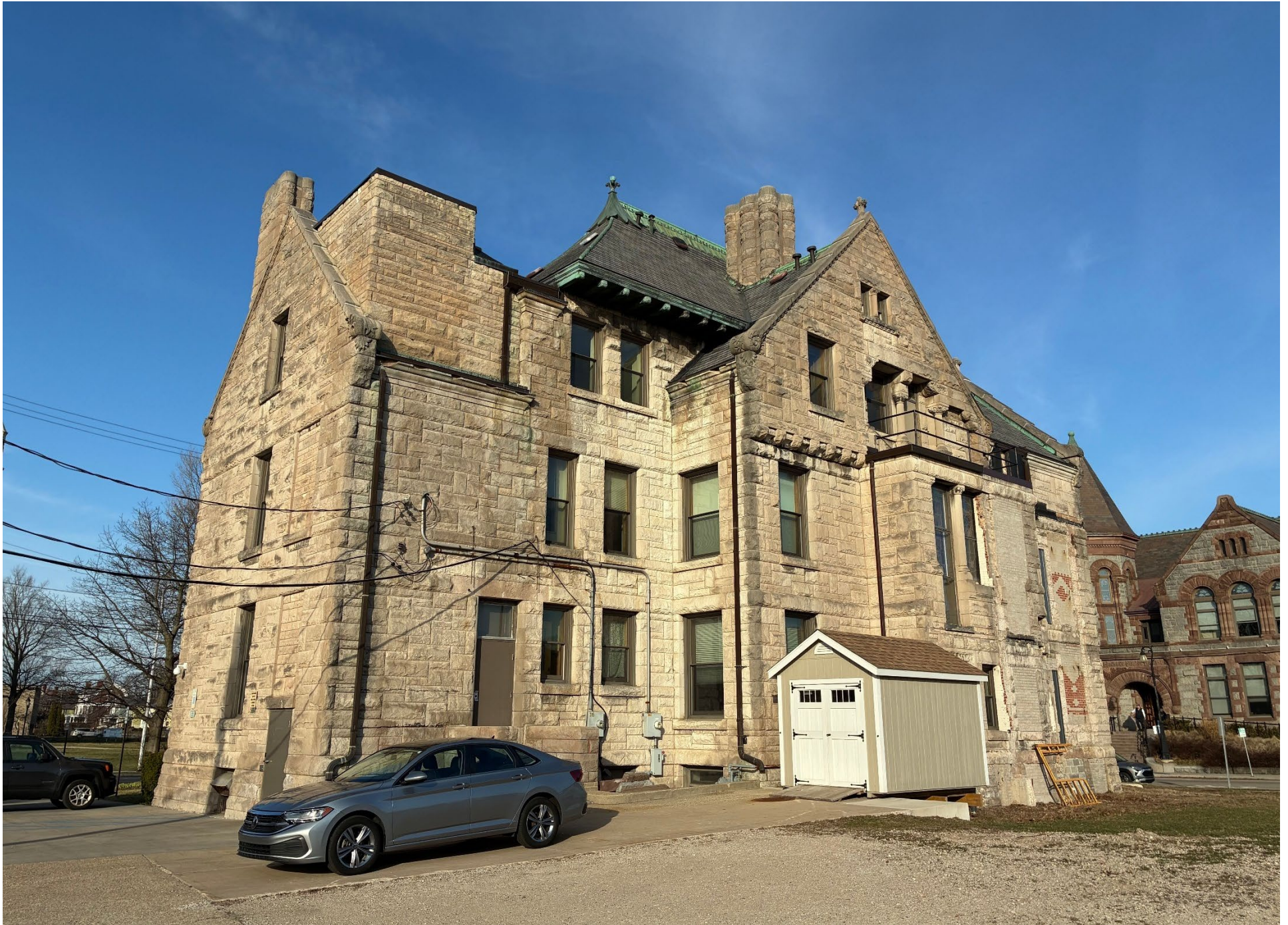
North elevation, looking northwest; proposed stair tower vestibule addition surrounds this corner of the building, roughly spanning the two visible doors.
