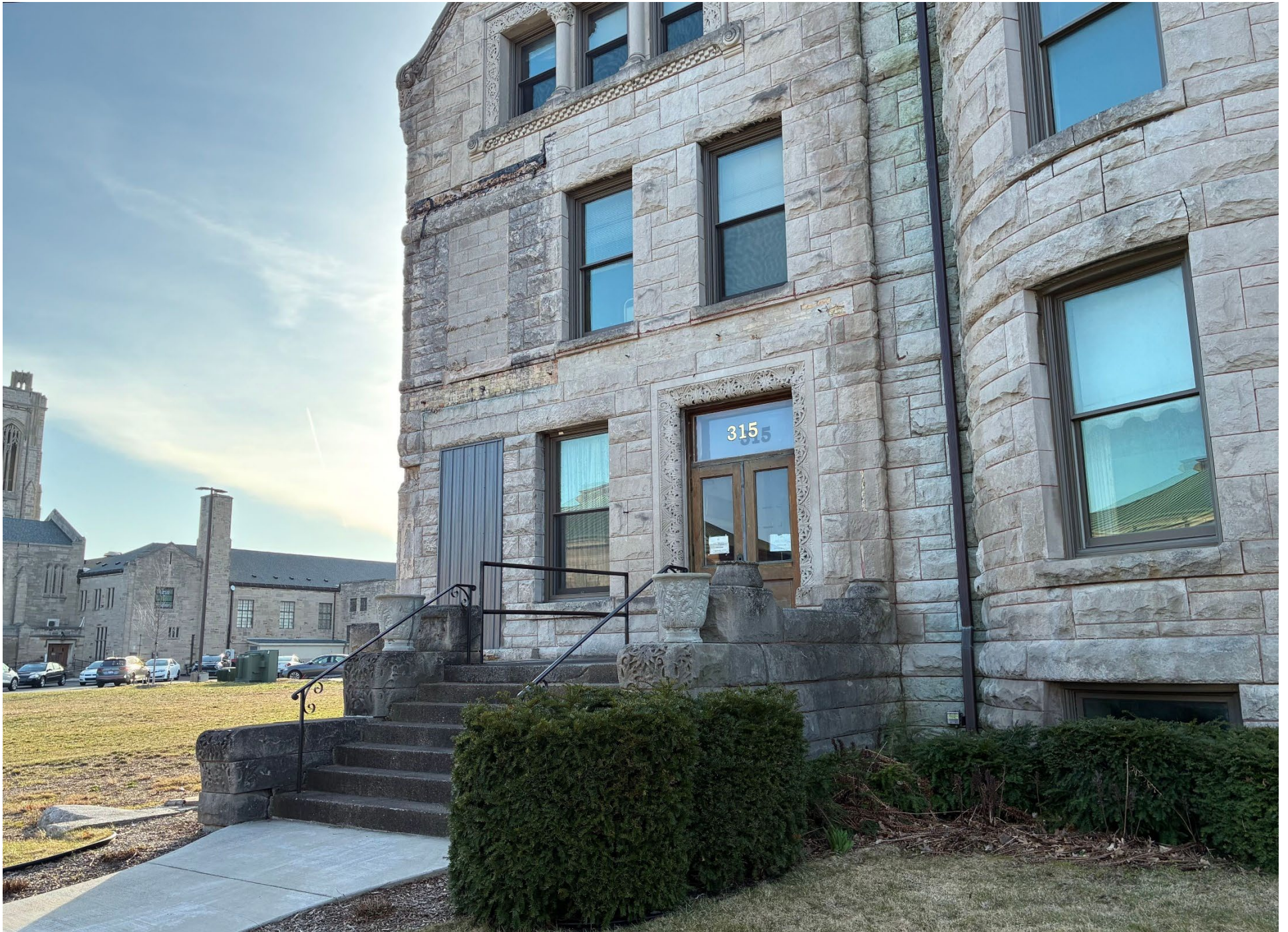
The remaining portion of the porch on the west elevation is proposed to be demolished and replaced with a new entry vestibule.
