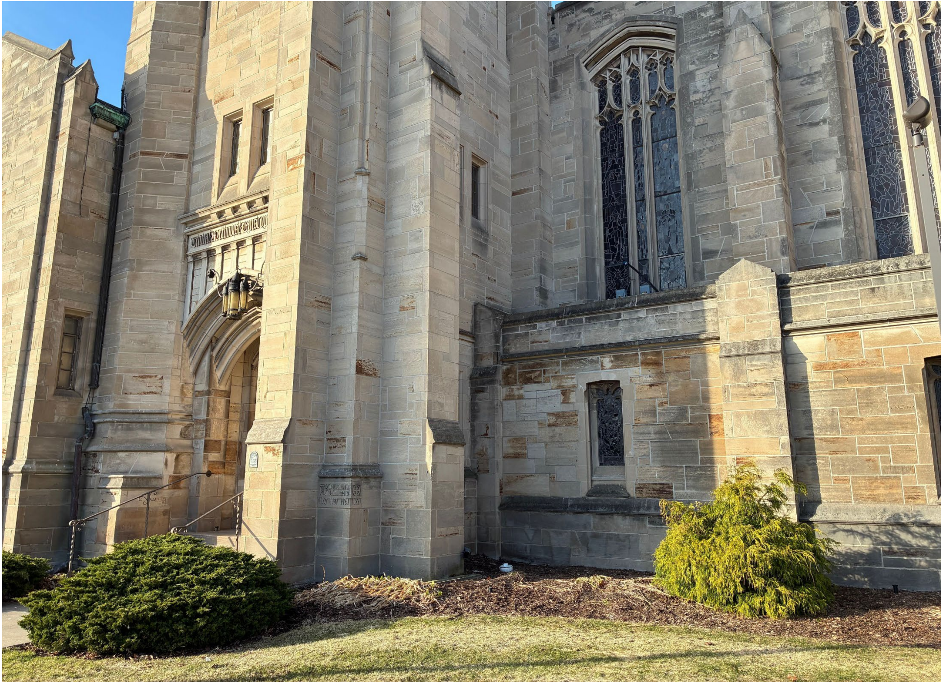
View of building from 2 nd Street, looking south; former location of roof-mounted unit with connection still visible at center.
