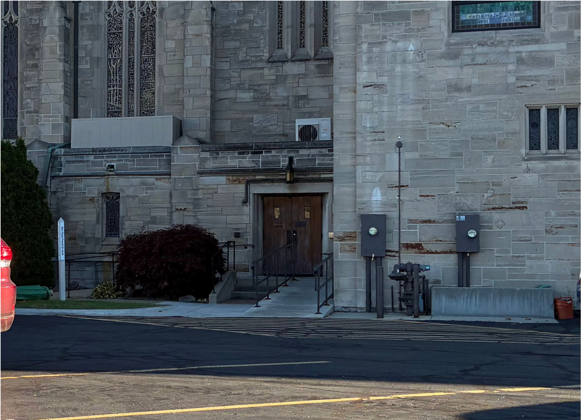
View of former roof-mounted unit with screen (left) from parking lot (photo from October, 2025).
