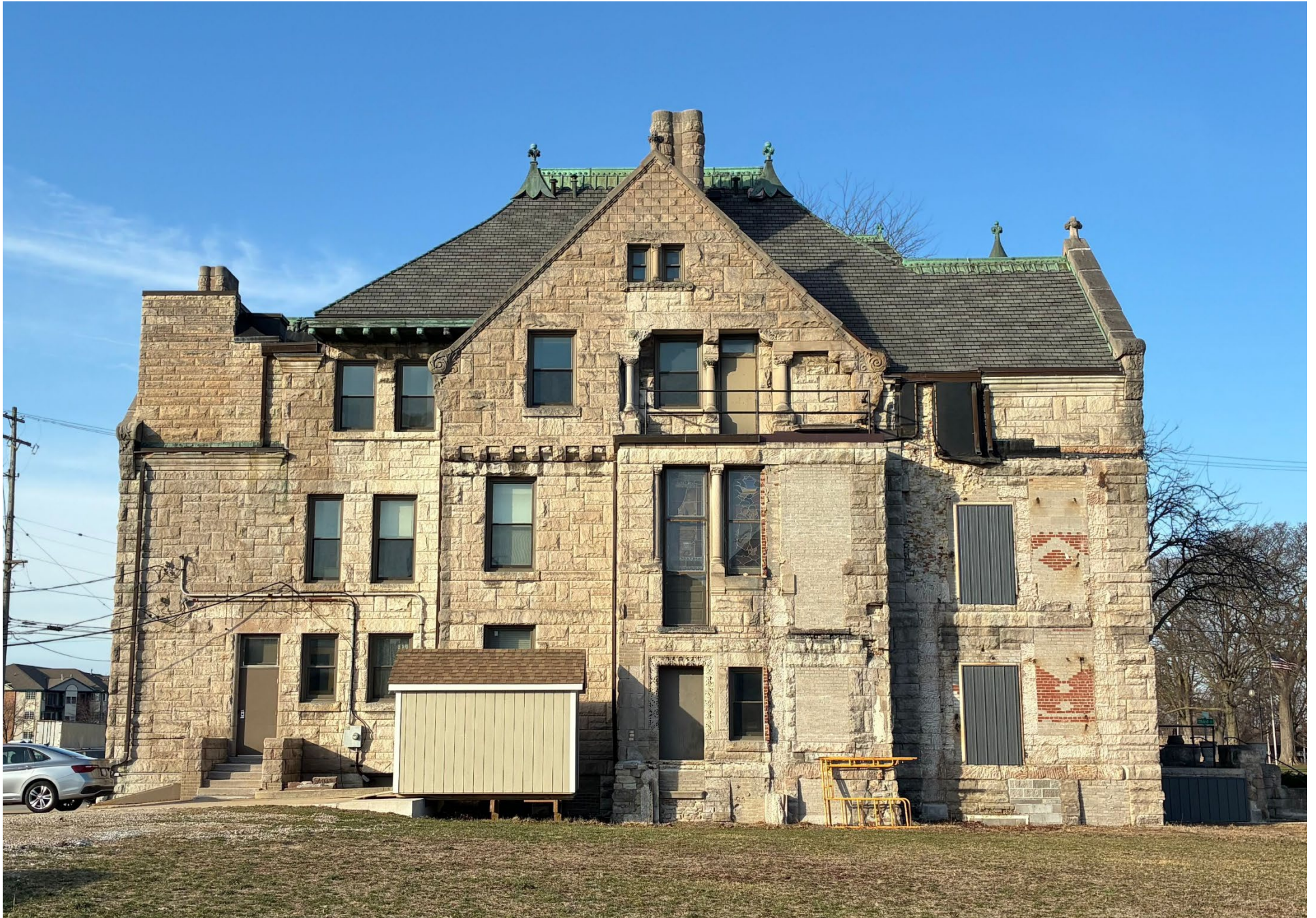
View of north elevation; visible at right (where the original window locations are bricked over and sheet metal covers former fire door openings from the 1950s addition) is the area where a decorative wall panel is proposed.
