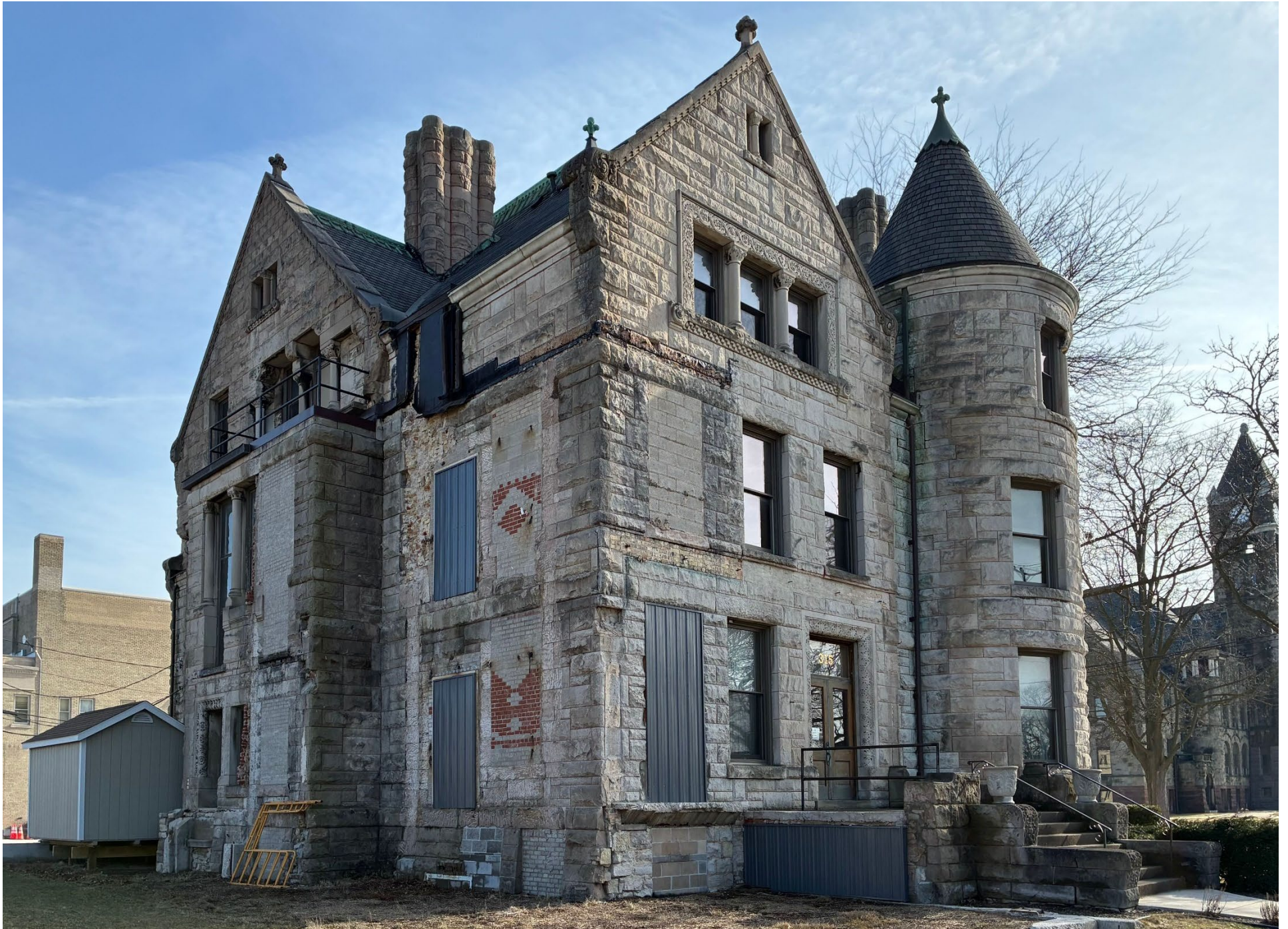
View of the west (facing W. Webster Avenue) and north (side) elevations from W. Webster Avenue, looking southwest.
