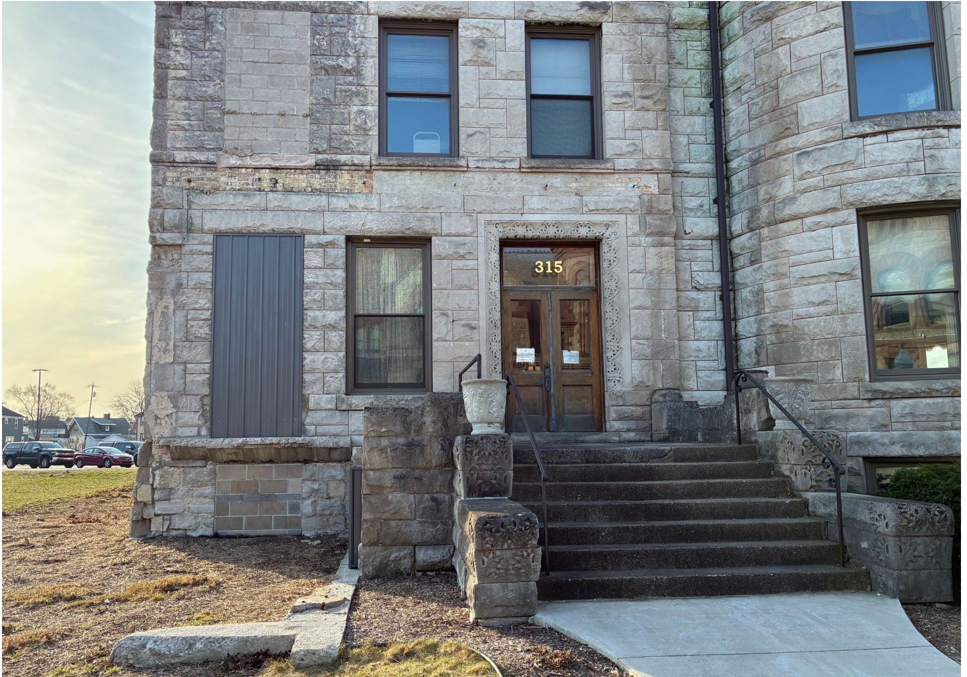
View of the remaining portion of the porch on the west elevation; the footing for the exterior wall of former building addition is visible at bottom, and the original porch roof's connection to the house is visible just below the second-floor window sills.
