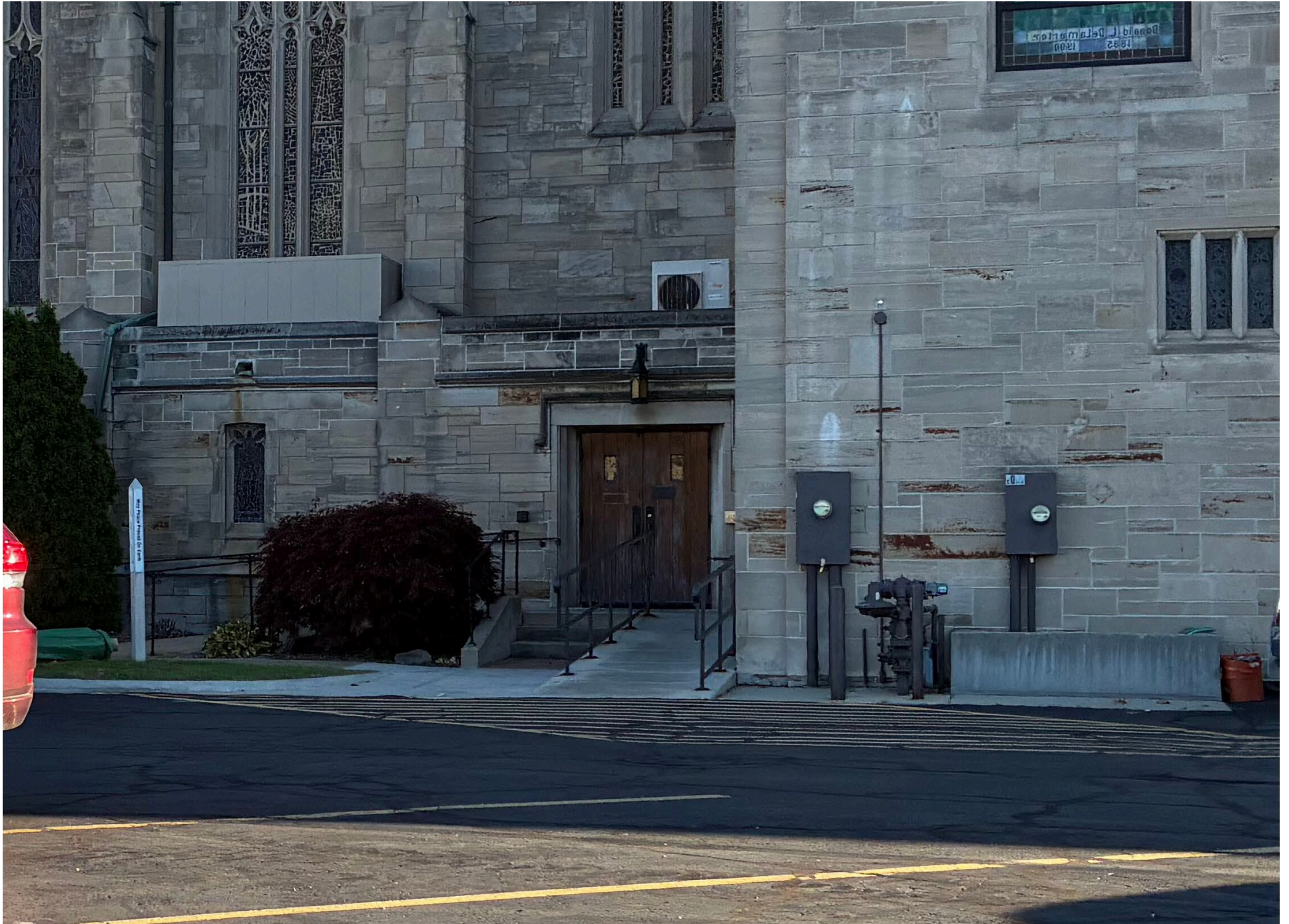
View of existing roof-mounted unit (right) and former screen (left) from parking lot (photo from October, 2025).
