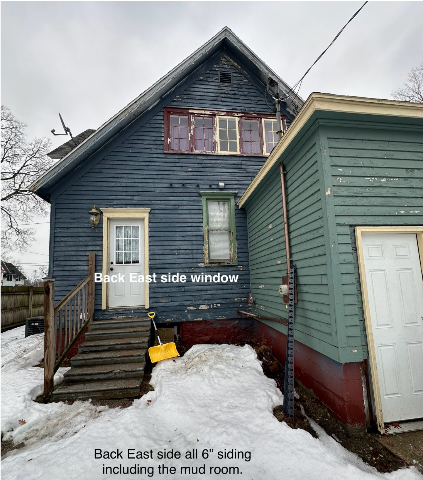
East (rear) elevation viewed from back yard with double hung window proposed to be replaced with casement visible at center.
