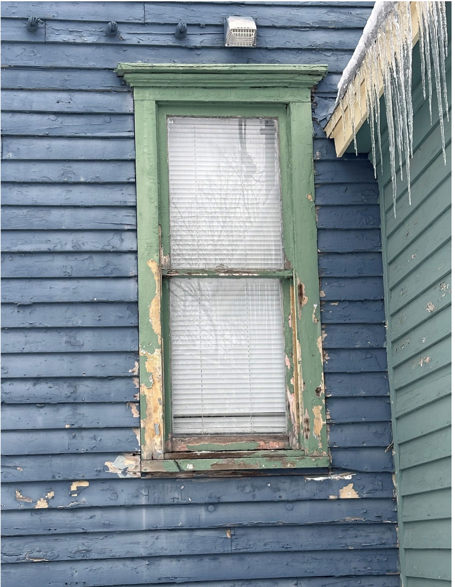
Detail view of window and siding on east elevation visible in previous photo.
