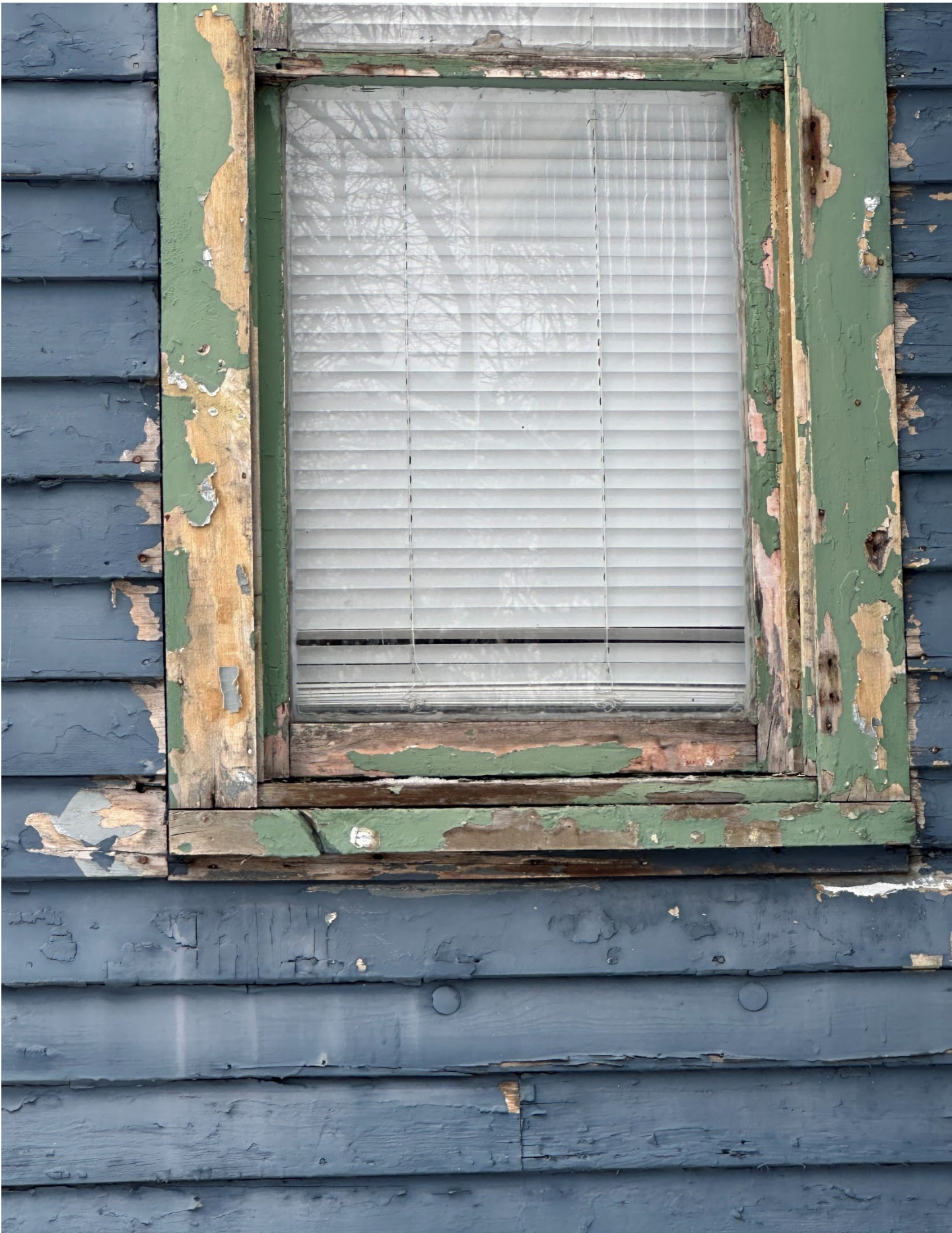
Second detail view of window and siding proposed to be replaced on east elevation.
