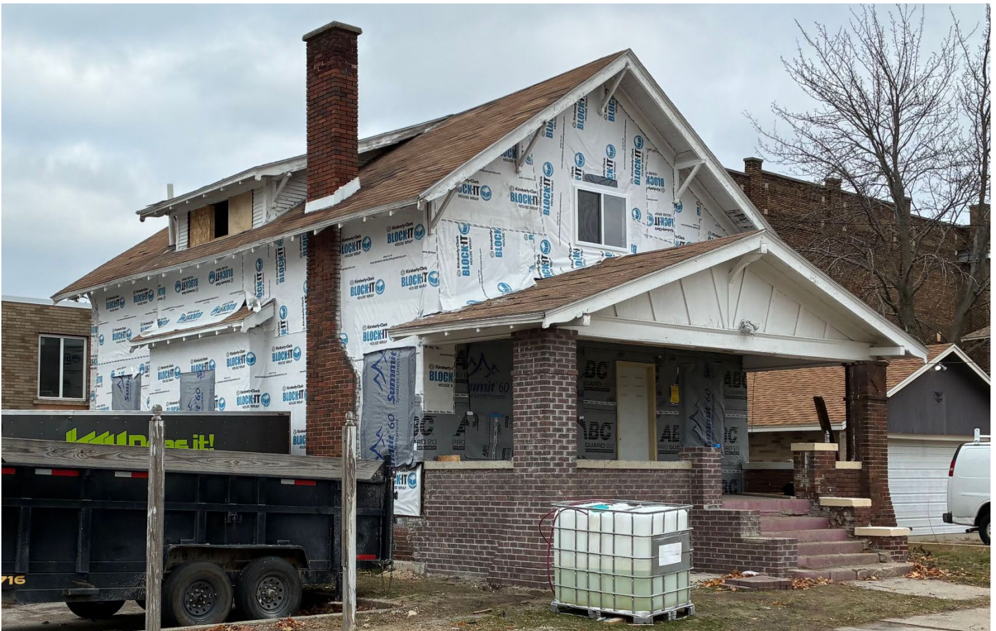
View of south (front) and west (side) elevations from Delaware (photo from November 2025).
