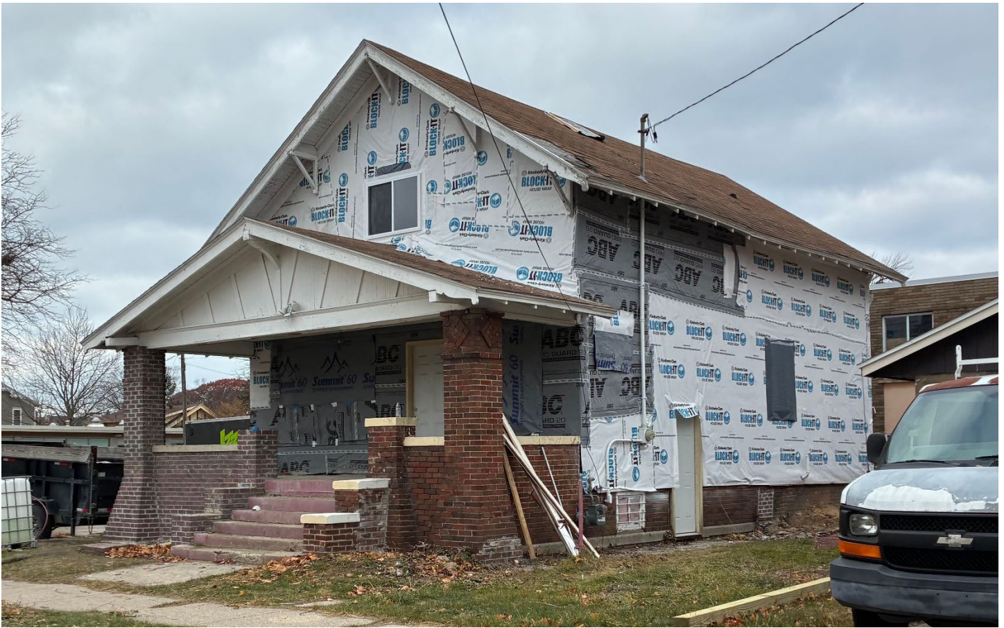
View of east (side) and south (front) elevations from Delaware (photo from November 2025).
