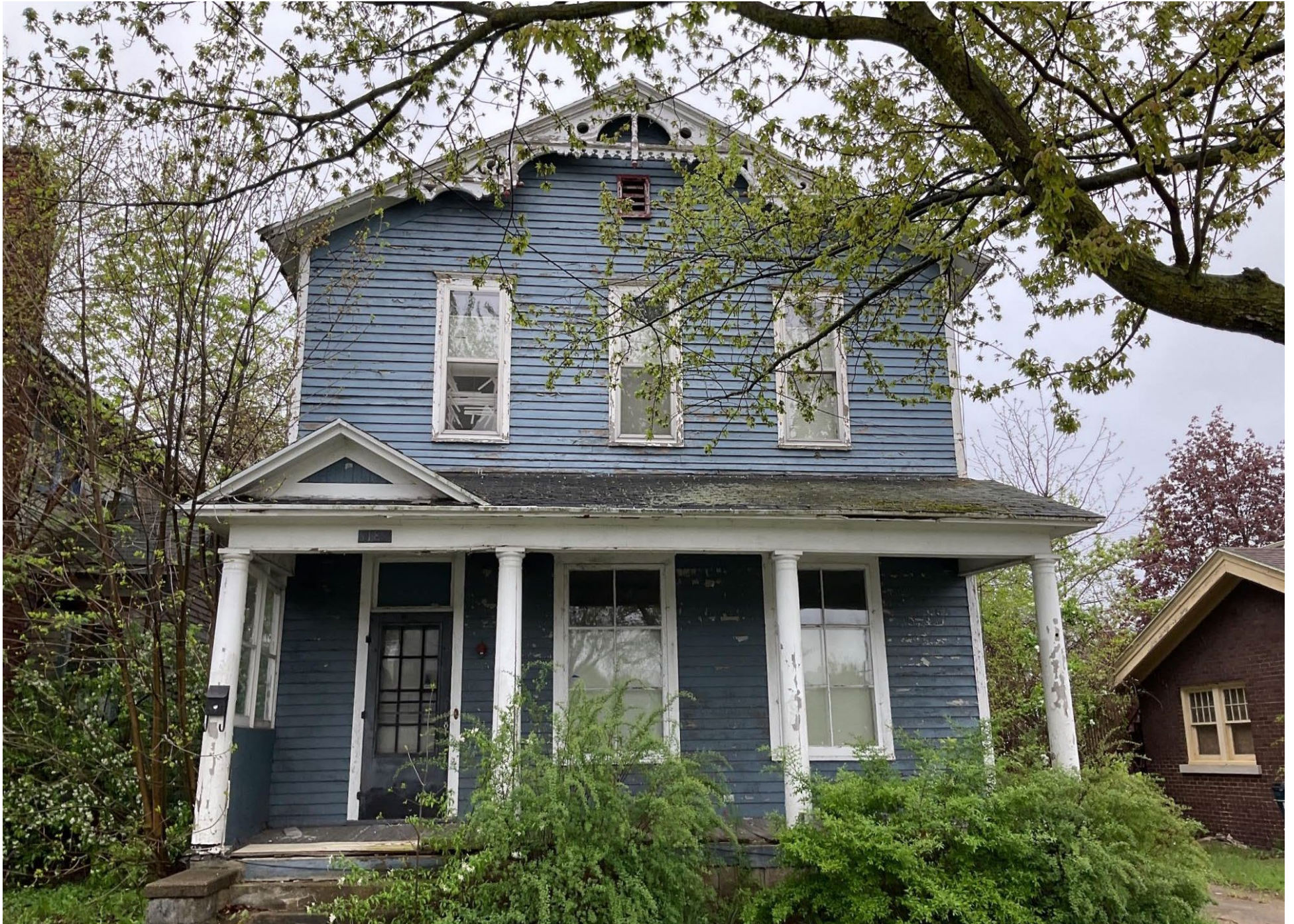
View of house from Ransom Street with former porch floor visible (photo from May 2024)
