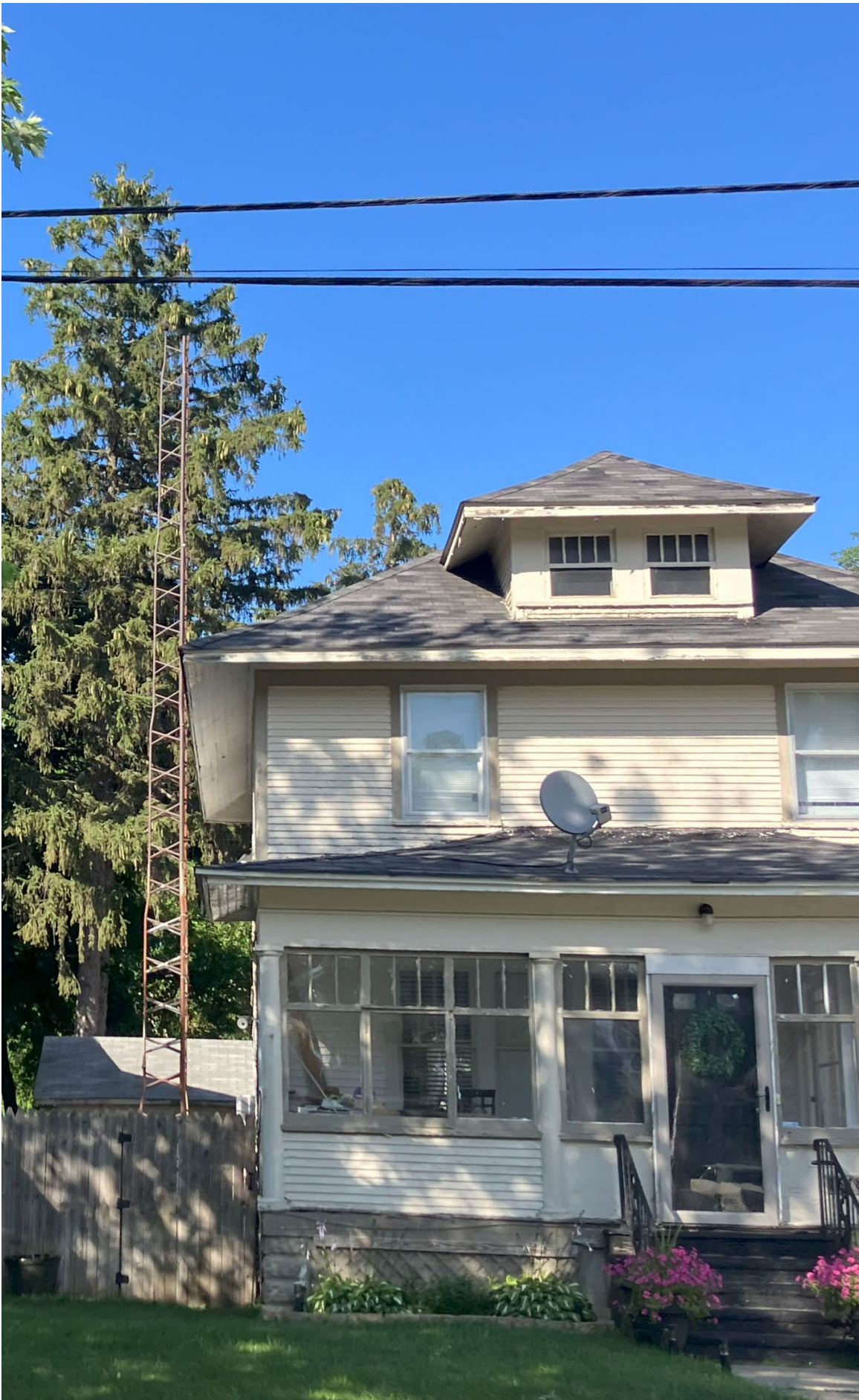
View showing original porch columns and windows, soffit, and trim (photo from June, 2024)
