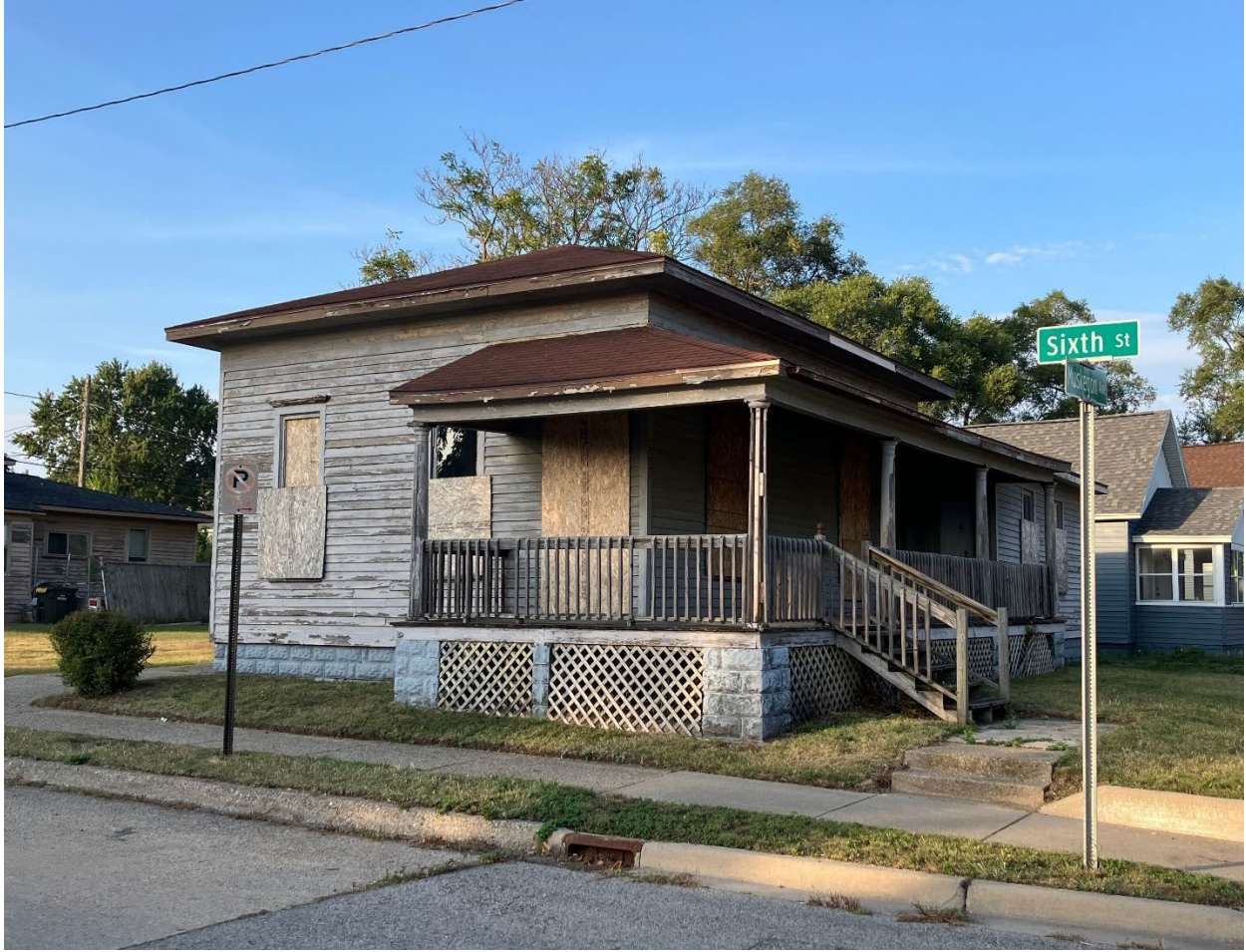
View of west elevation from 6 th Street with front door (boarded) and two windows to be replaced
