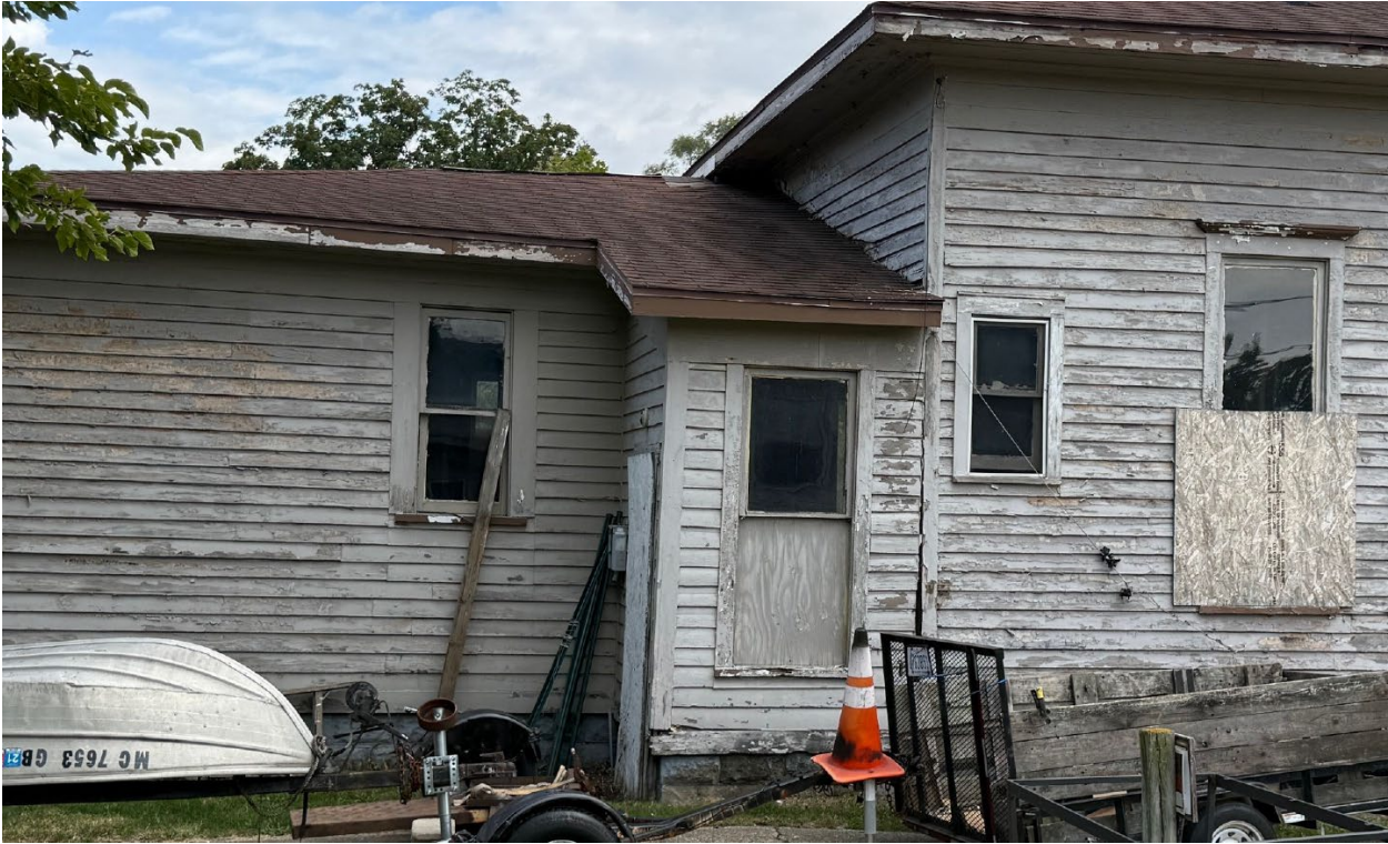
Leftmost window on north elevation to be replaced with a 36"x80" door, exterior steps, and landing
