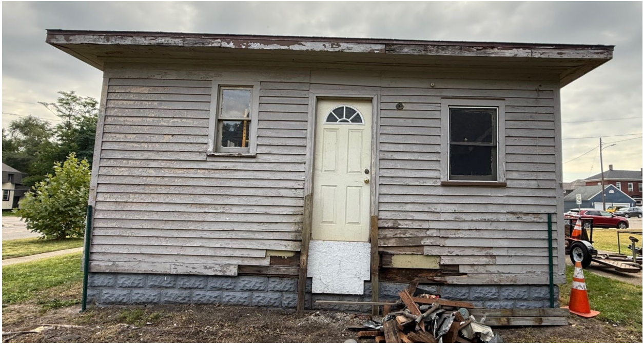
Two windows and one of two doors on the east elevation to be removed
