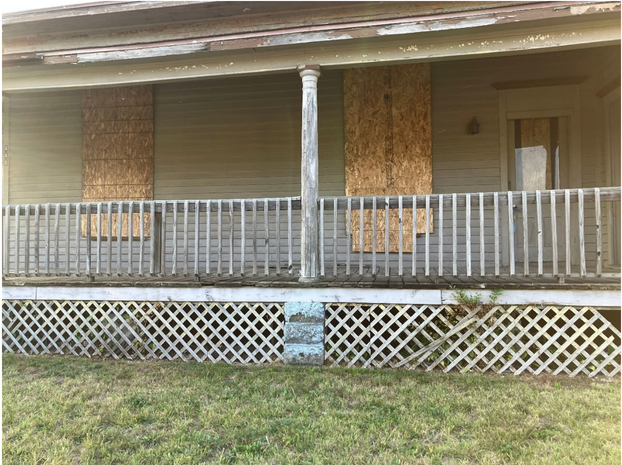
Two doors on front porch visible at right to be removed, and two boarded windows to be replaced
