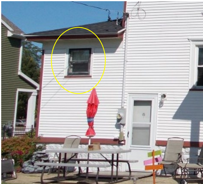
Rear window prior to replacement (photo from June 2017)
