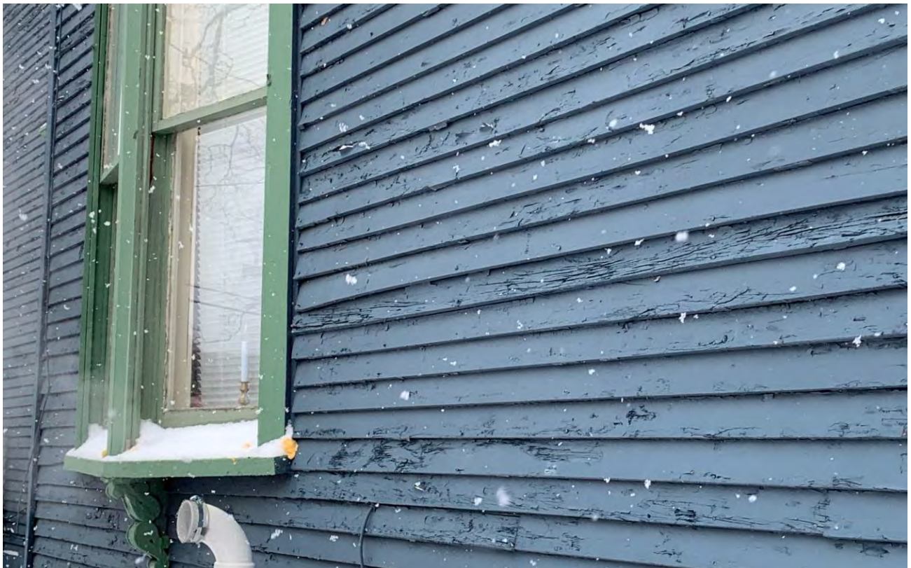
Examples of deteriorated wood siding on the house.
