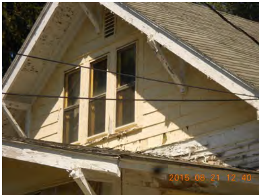
Exposed wood siding/deterioration.
