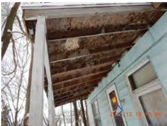
Exposed wood under roofing of front porch.
