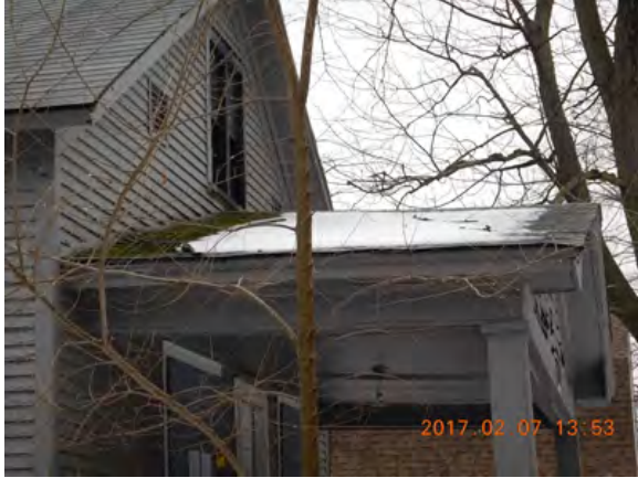
Roof deteriorated above porch.
