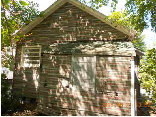
Rear of structure – deterioration.
