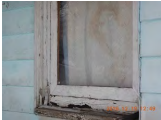
Rotted/exposed wood around windows.
