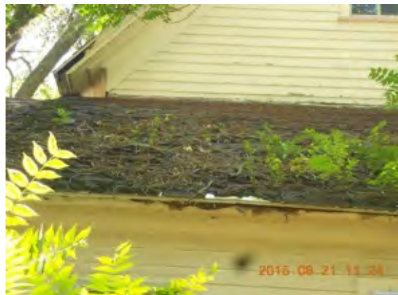
Roofing is deteriorated.
