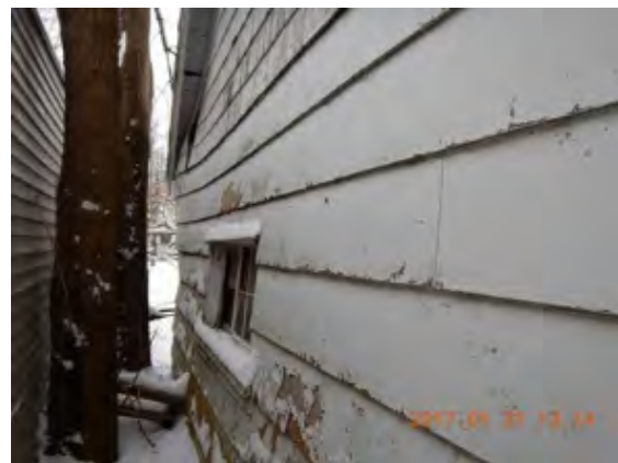
Garage wall is bowing out.
