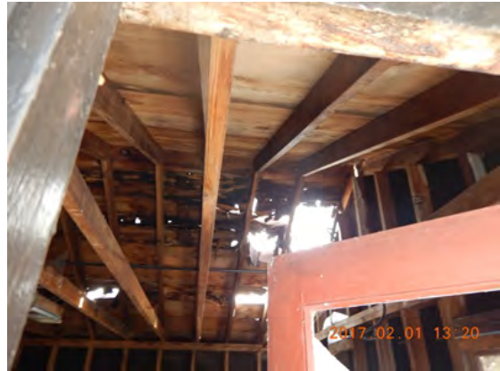
Hole in roof of garage.
