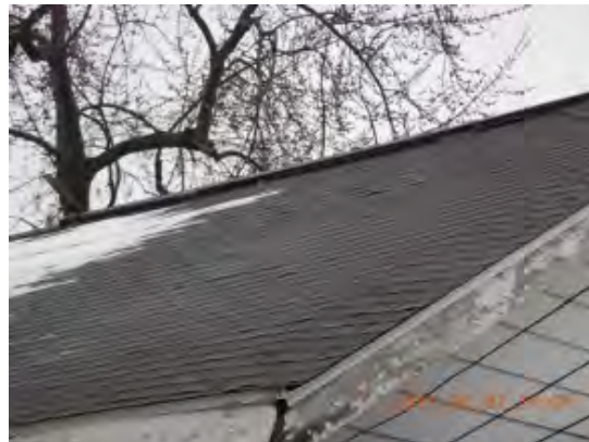
Roof bowing & deteriorated.
