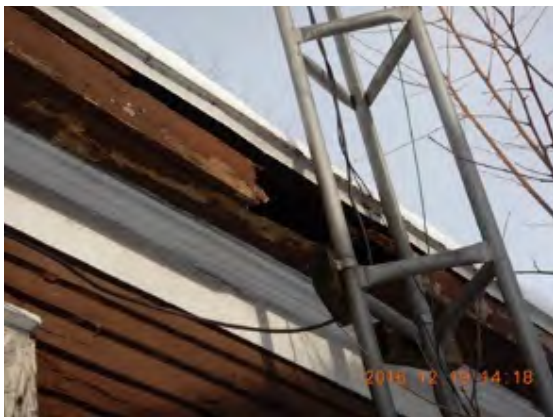
Eaves/faschia rotted & holy.
