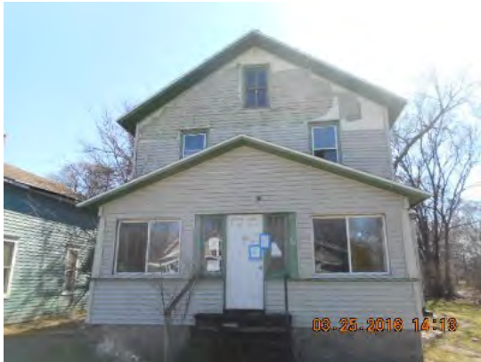
Front-siding falling off throughout.
