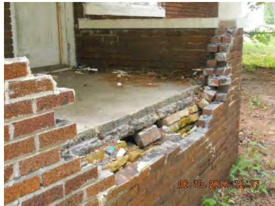
Side porch bricks deteriorated.
