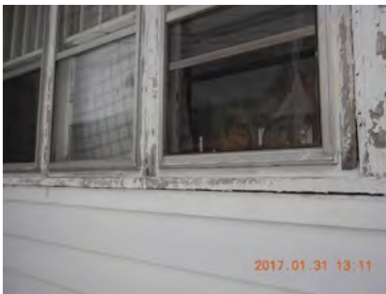
Window frames-rotted & peeling paint.
