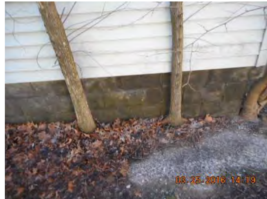
Trees growing from foundation-damaged.
