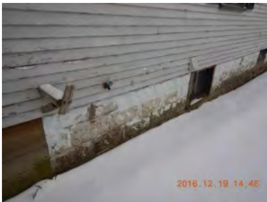
Foundation is bowing.
