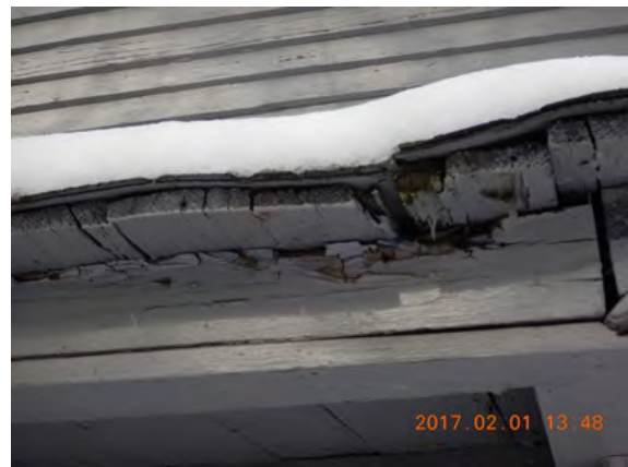
Rotted wood under roofing.
