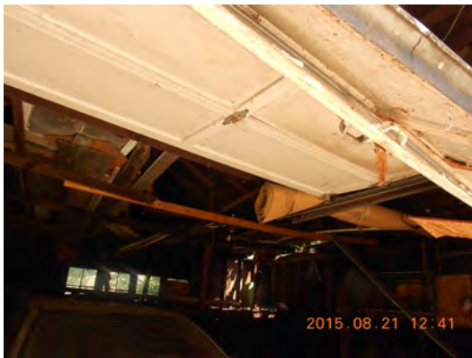
Interior garage holes in roof/sides
