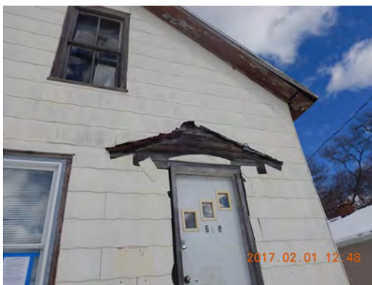
Rotted/exposed wood above front door.
