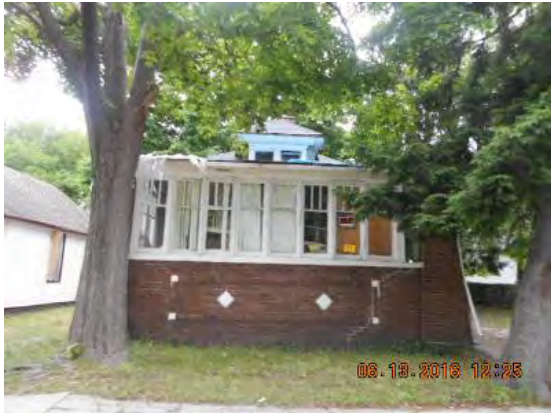
Front of home-roof failing.
