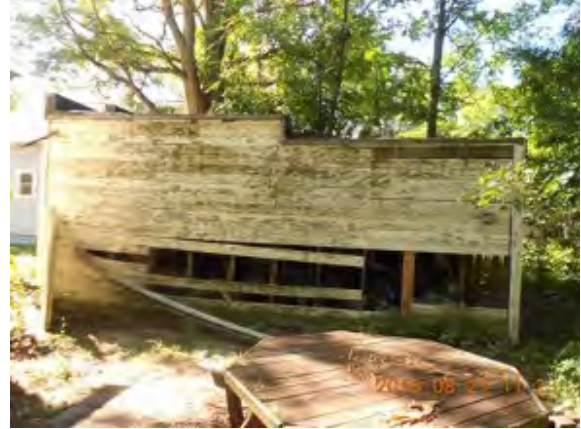
Garage-side wood is missing/falling off.
