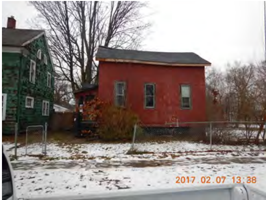
Front & sagging roof.
