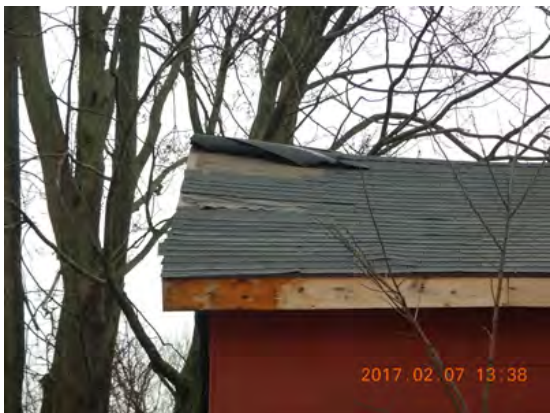
Roofing deteriorated & falling off.
