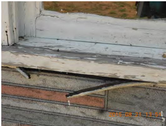
Rotted window sealing.
