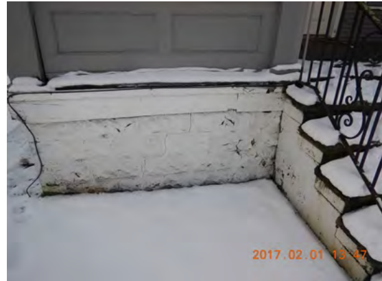
Large cracks in foundation.
