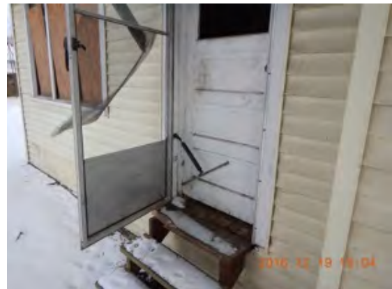
Wood under door leading into house is rotted & exposed to weather.
