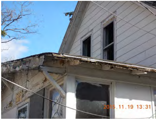
Deteriorated/rotted wood at front porch.
