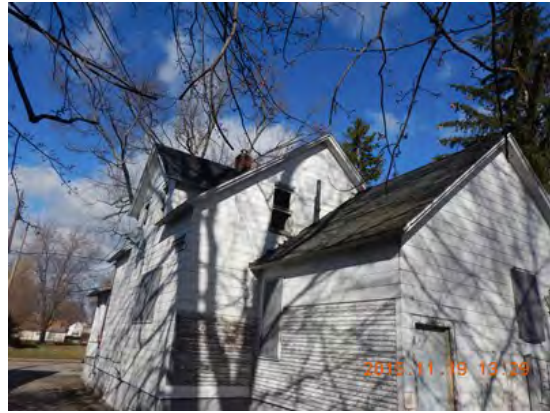
Side/rear missing siding.
