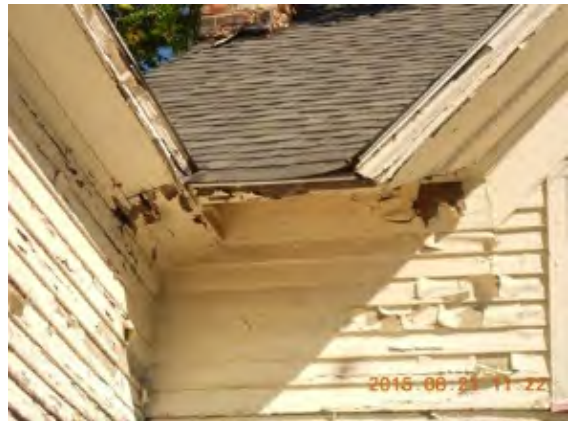
Wood exposed & roofing area deteriorated.
