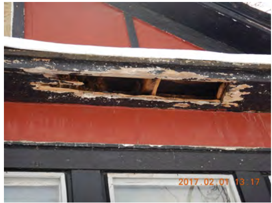
Holy wood in eaves/fascia.
