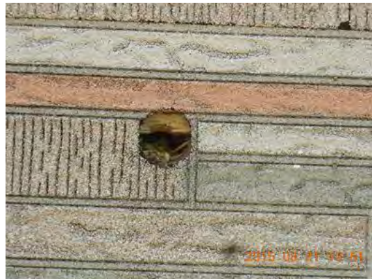
Holes in siding throughout.
