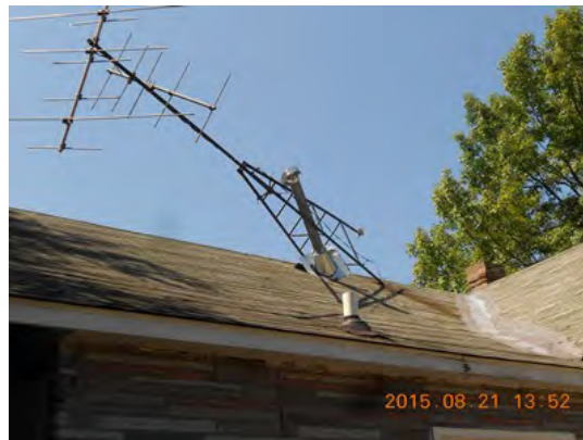
Roofing is damaged.
