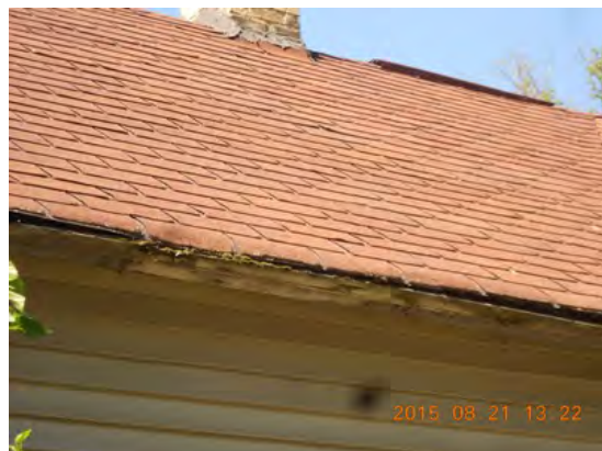
Deteriorated roofing & rotted wood under.
