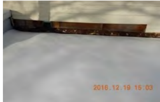
Siding missing-wood exposed.
