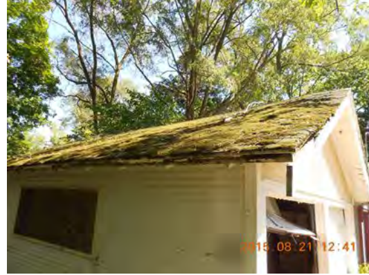
Garage roof rotted.
