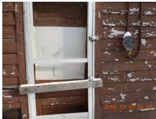
Wood exposed due to peeling paint.
