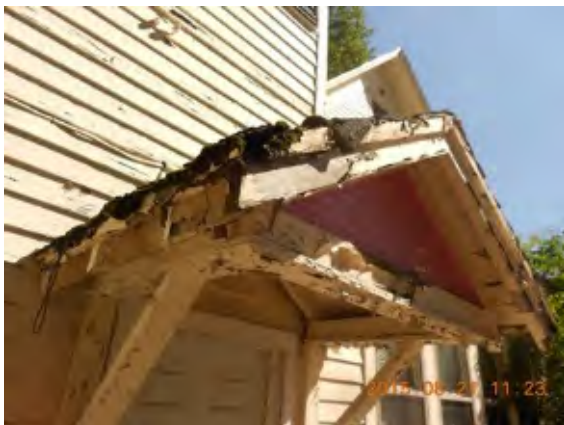
Wood exposed/rotted/peeling paint.
