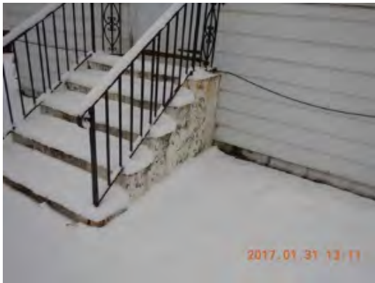
Foundation cracked/missing mortar.
