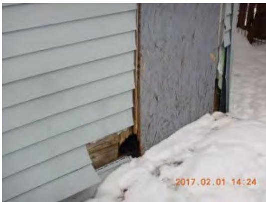
Holes in wood & siding.
