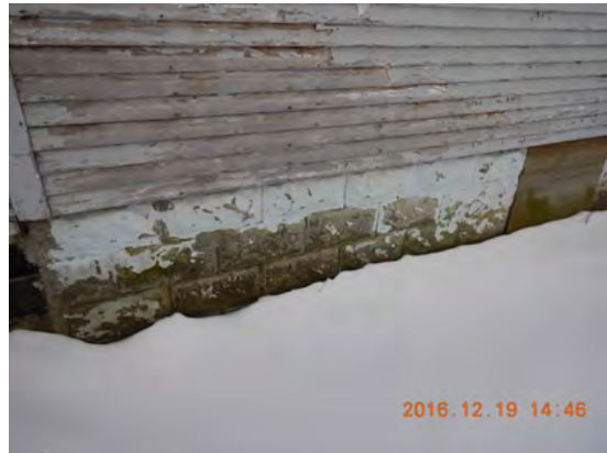
Foundation has cracks & missing mortar.
