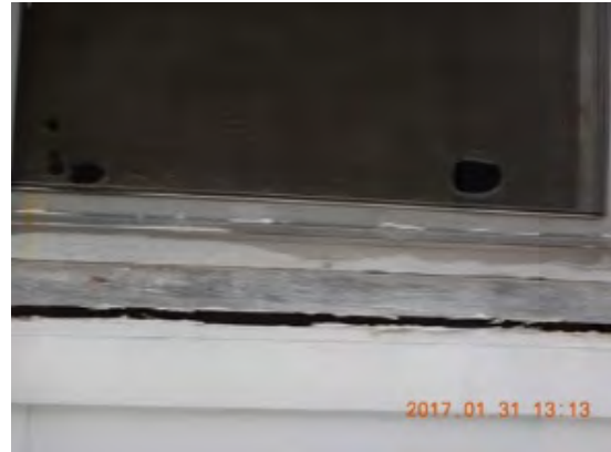
Windows are not sealed & wood rotted.
