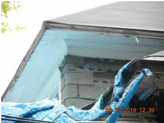
Roofing has no shingles.
