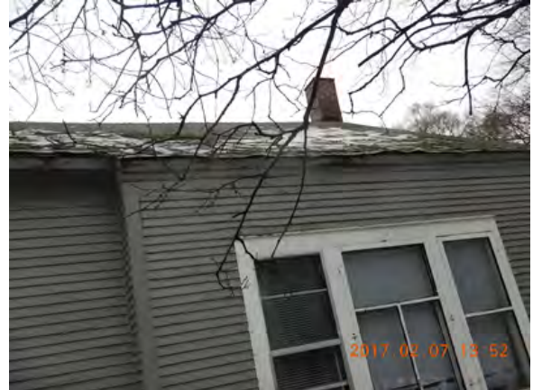
Roof is deteriorated/missing shingles throughout.
