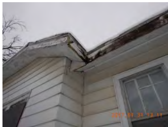
Rotted wood in fascia & eaves.
