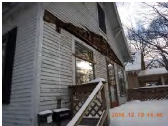
Front porch-wood exposed & rotted.
