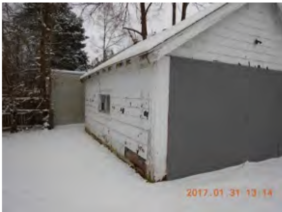
Garage has exposed wood & peeling paint.
