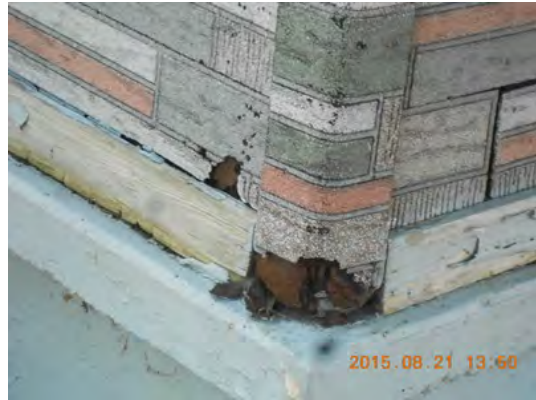
Rotted/missing siding—throughout exterior.
