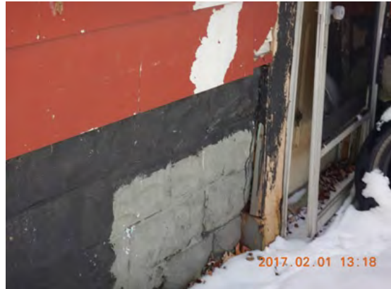
Foundation-separating from doorway.
