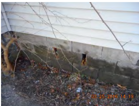
Foundation has holes/cracks/bowing.
