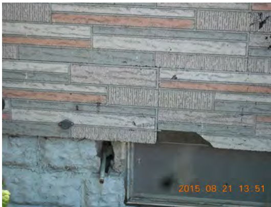
Hole in foundation.
