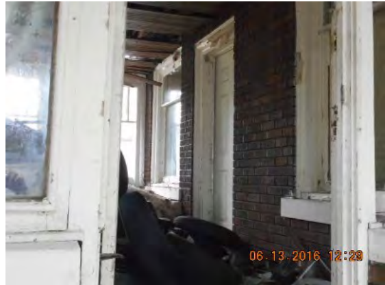
Front porch interior roof falling.
