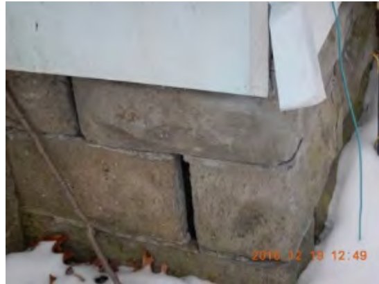
Foundation missing mortar.
