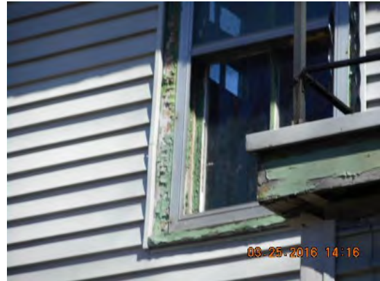
Window improperly sealed & wood rotting.
