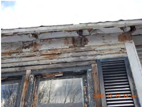
Rotted/exposed wood & peeling paint.
