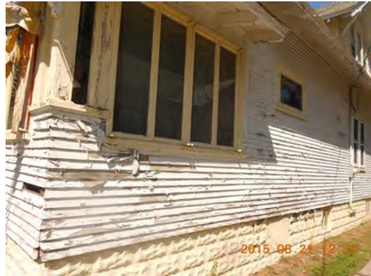
Peeling paint/rotted wood.
