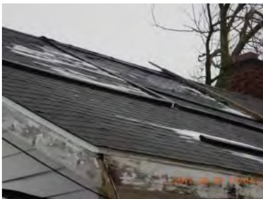
Roof bowing & deteriorated.
