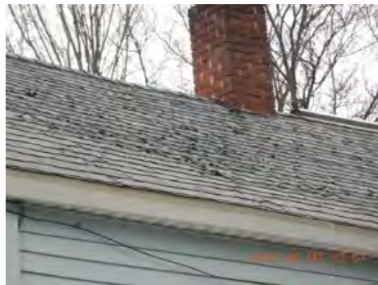
Roof deteriorated throughout.
