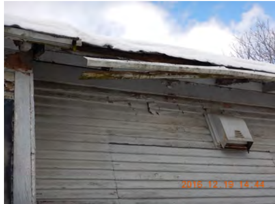
Roofing area rotted (multiple areas).
