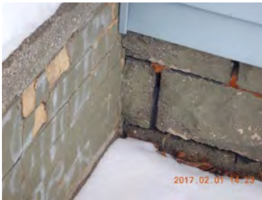
Foundation-missing mortar throughout.
