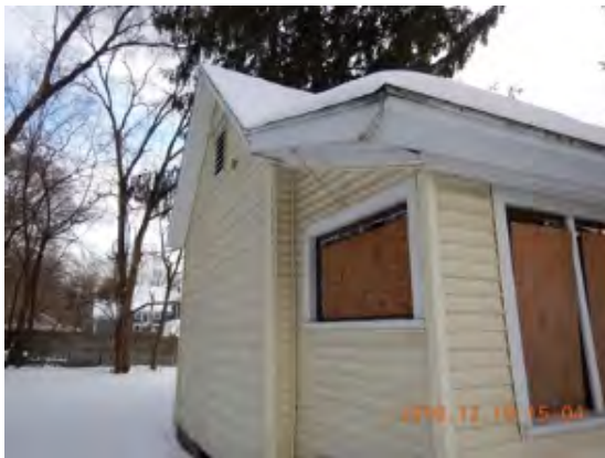
Roofing is buckling up & boarded windows leave exposure to the interior.
