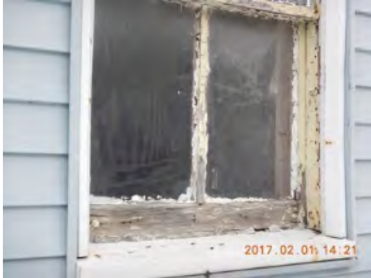
Windows-rotted wood throughout.
