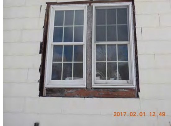
Many areas appear to have new windows. No permits were found. Wood rotting.
