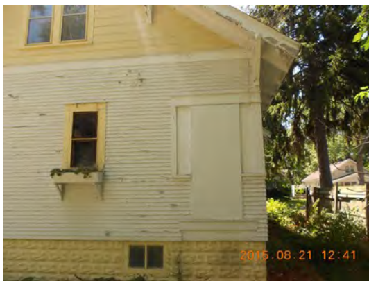
Cracked foundation. Boarded side door with no steps.
