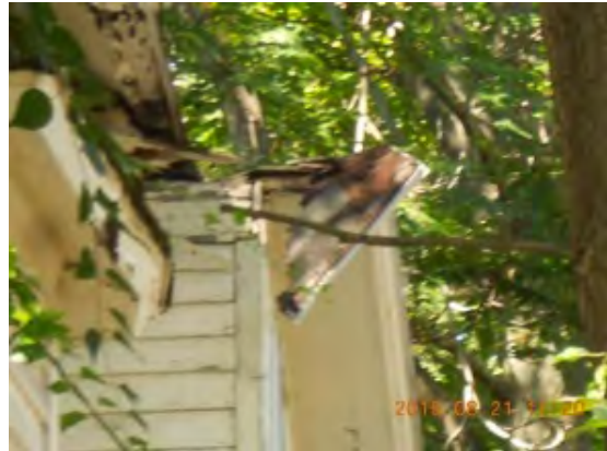
Rotted/broken eaves & fascia.
