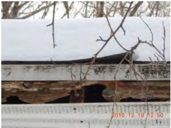
Rotted/holy wood in eaves/fascia.
