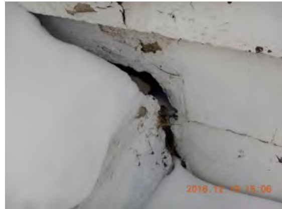
Foundation cracked & caving in.
