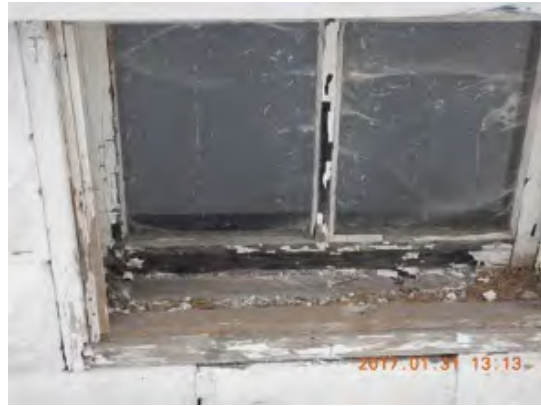
Basement window-foundation deteriorated.
