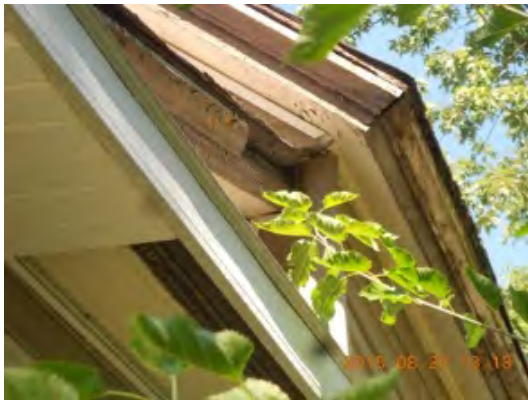
Wood rotting under the roof.
