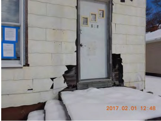
Wood exposed where siding is falling.
