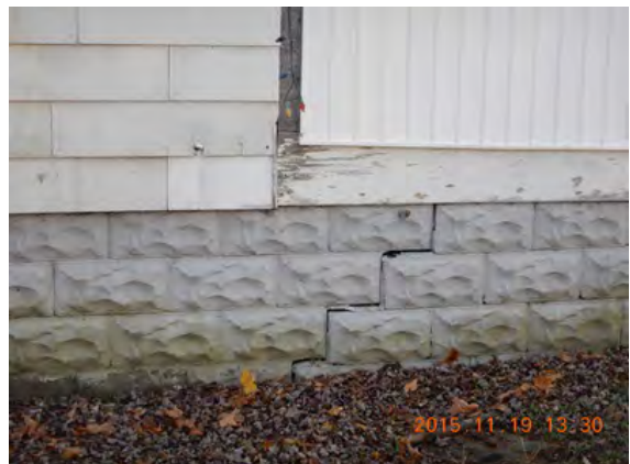
Siding has cracks throughout.
