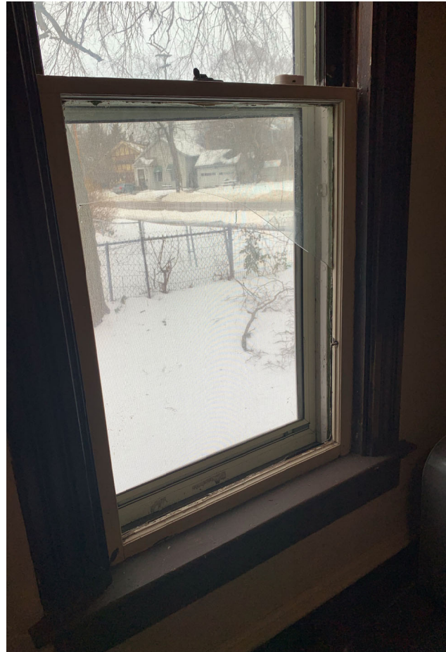
Interior view of same window with broken glass
