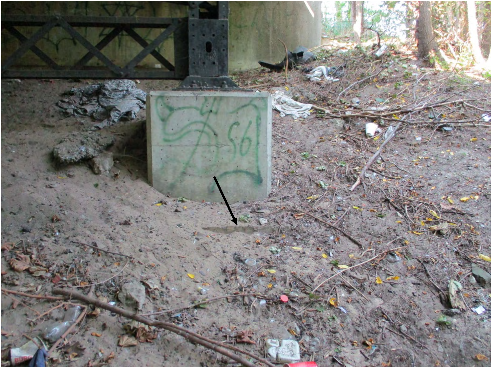
Pier 1W north support has exposed footing.
