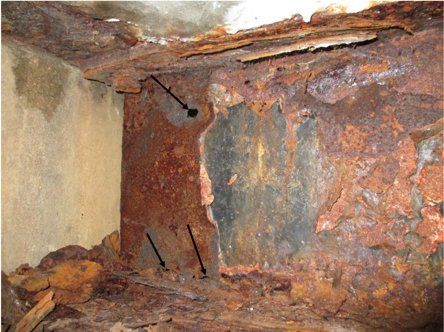
Beam 5S holes have formed under heavy pack rust
