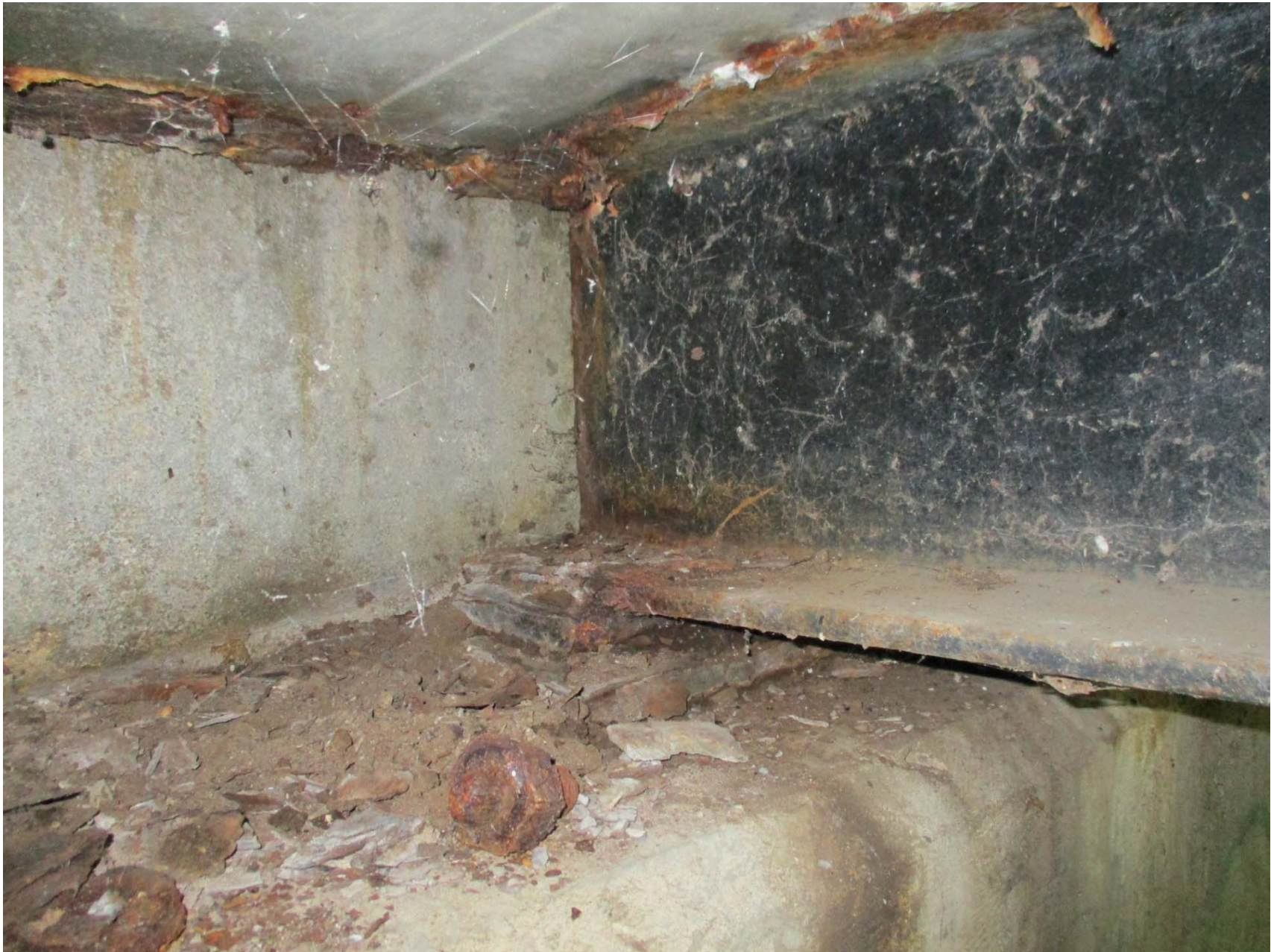
North fascia at west abutment, sheared off anchor bolt
