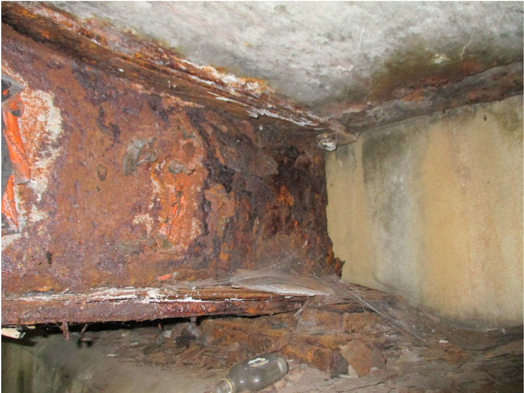
Joint leakage causing heavy corrosion to beam ends, beam 5S
