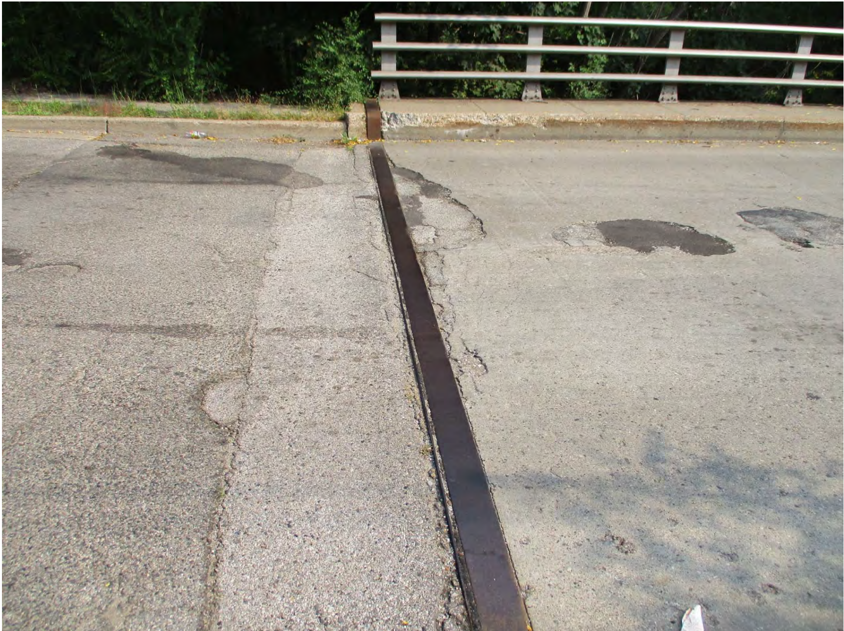
West expansion joint with spalled deck end in WB lane
