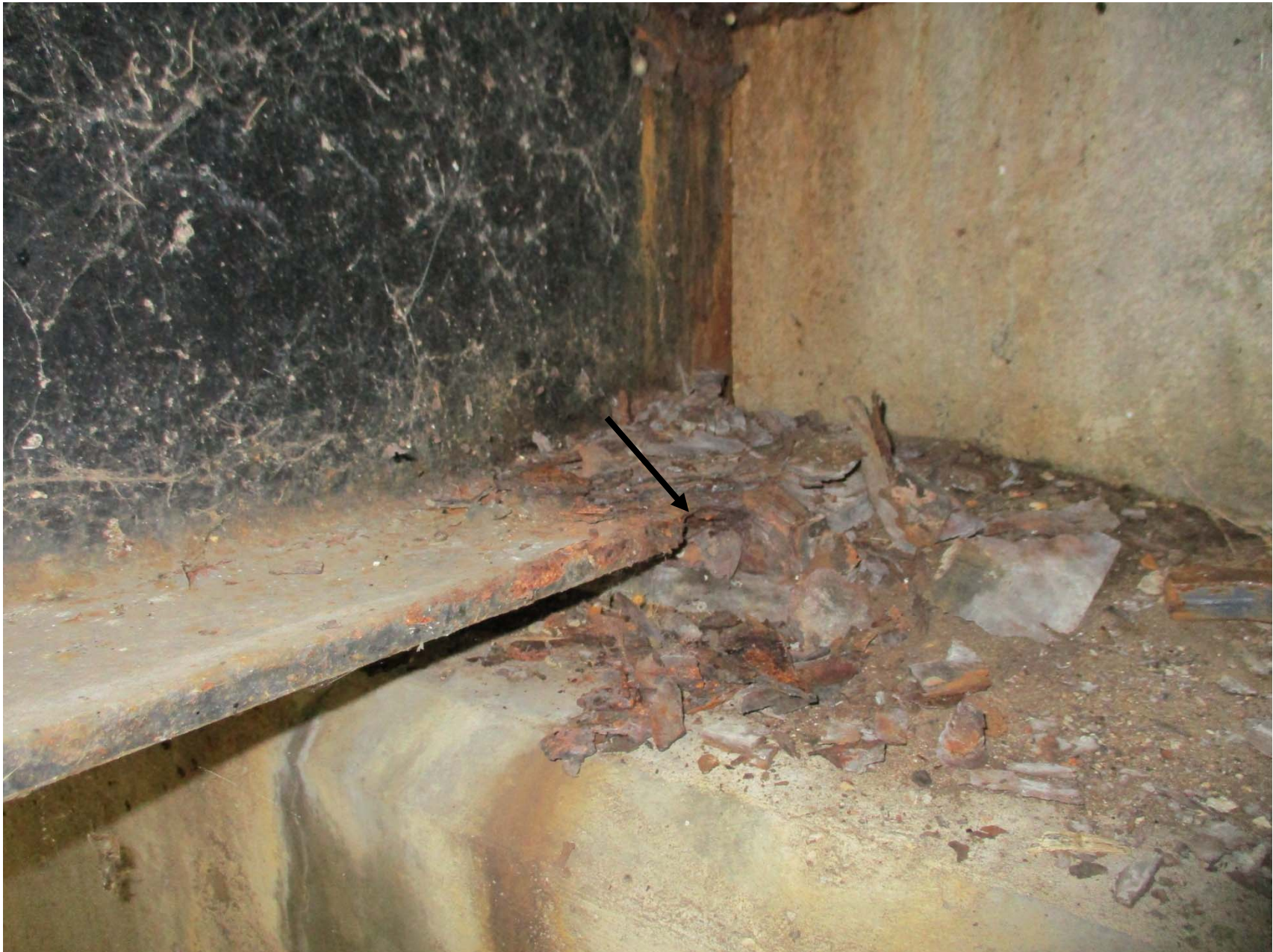
Section loss to east end of north fascia bottom flange and anchor bolt
