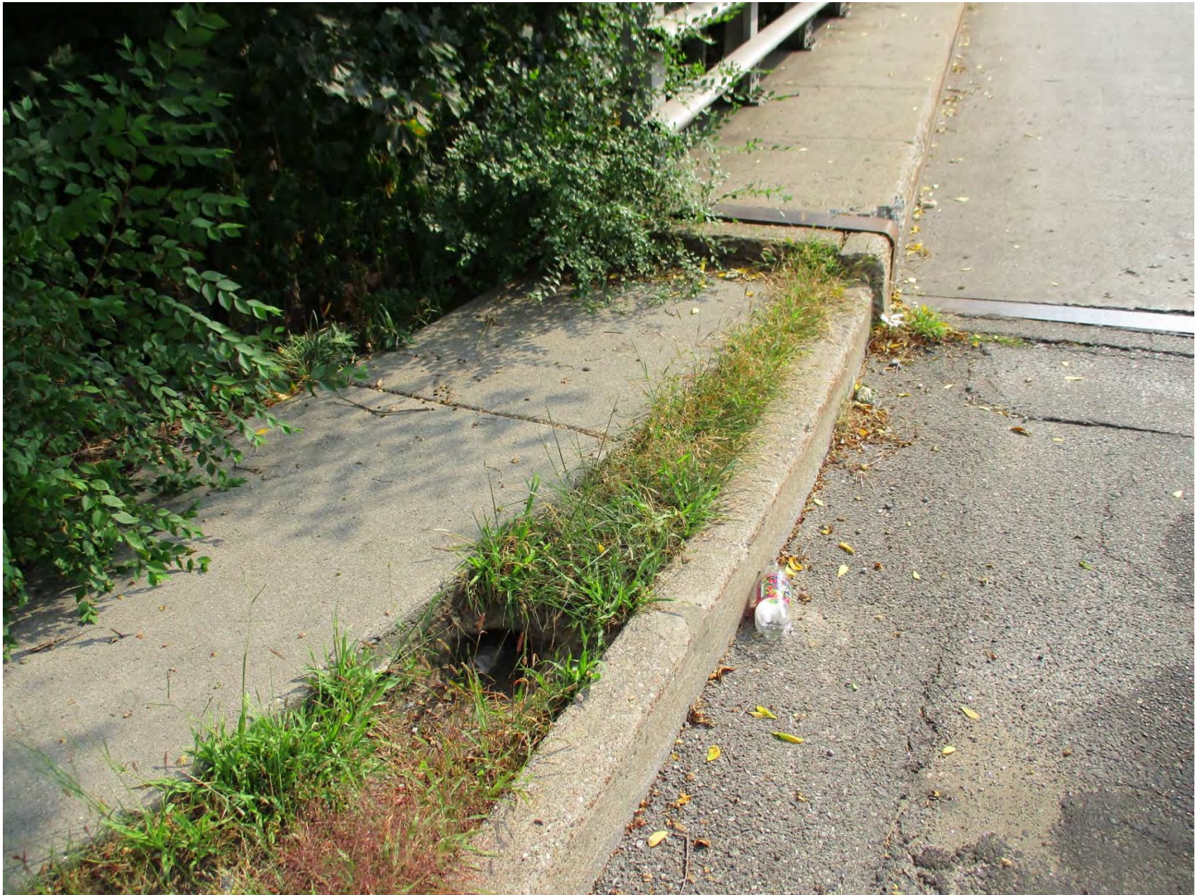
Animal hole under NW sidewalk, settlement at the bridge sidewalk where the retaining wall sheets failing
