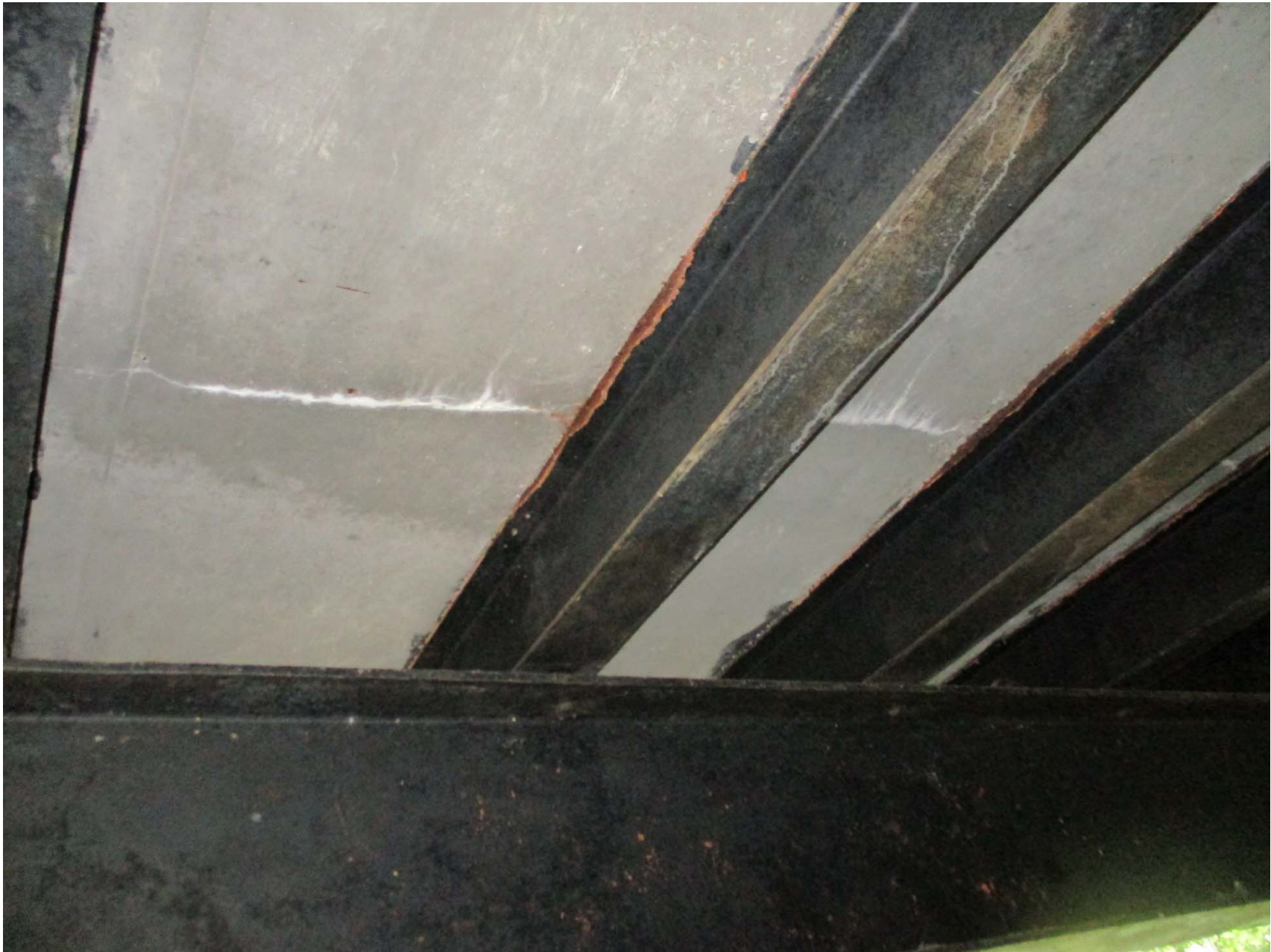
Full depth deck cracks with efflorescence, causing rust on beam flanges
