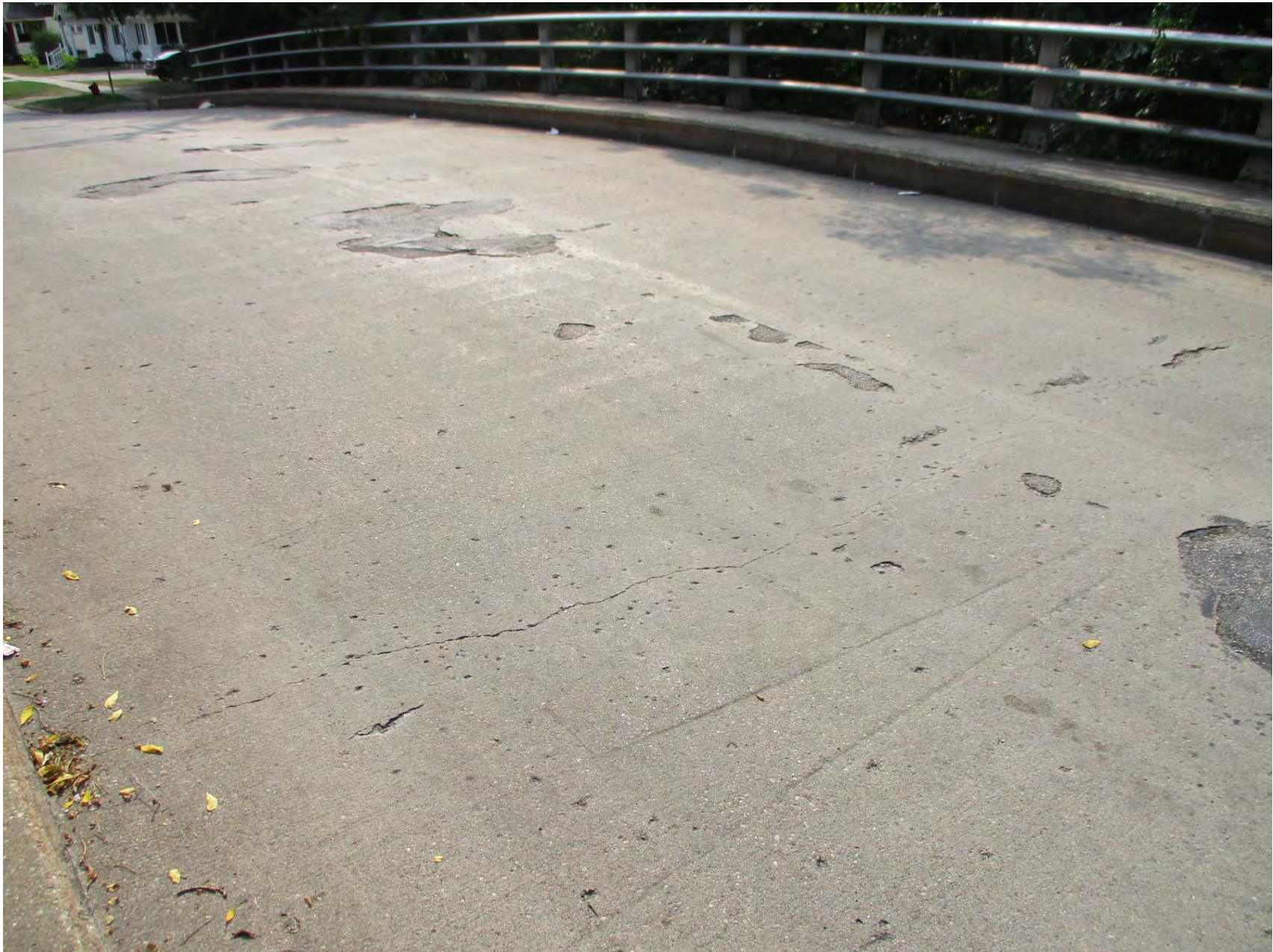
Many full depth transverse cracks in the deck. Spalling, patches, and delamination along center 1/3 rd of deck
