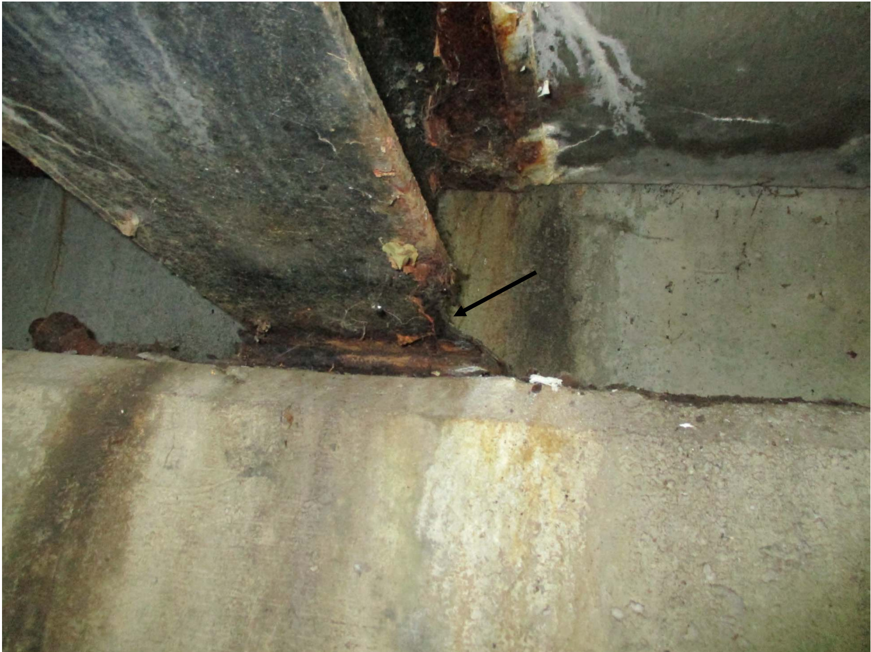
Full section loss along edge of bottom flange, north fascia at west abutment
