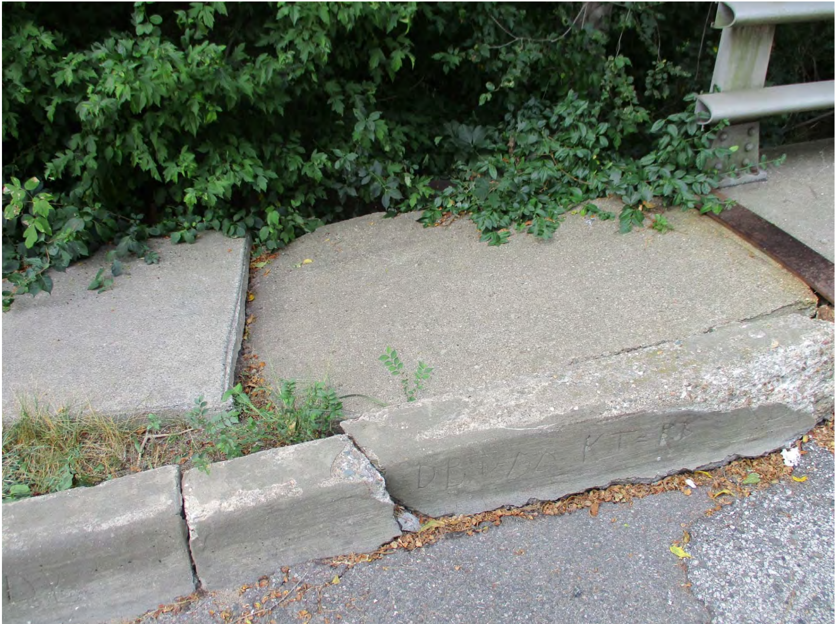
Retaining wall sheets failing the SE quadrant leading to sidewalk and curb settlement
