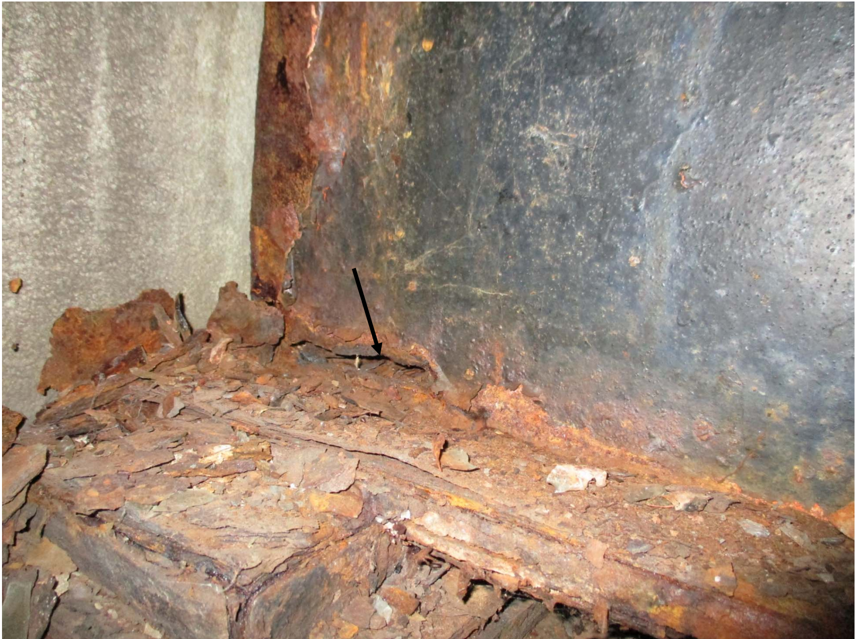
Beam 3S west end, hole along bottom of web
