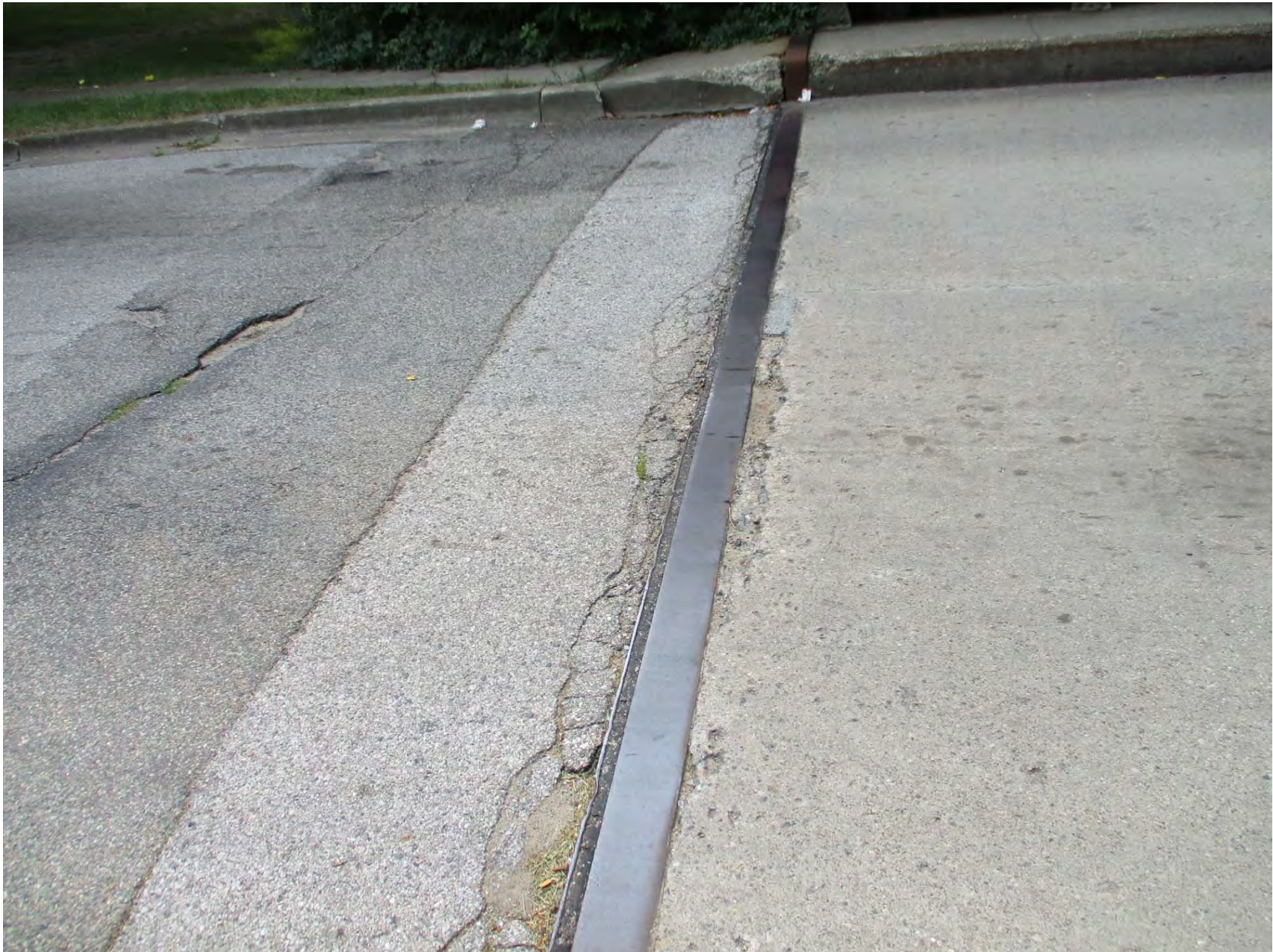
Spalling along east expansion joint
