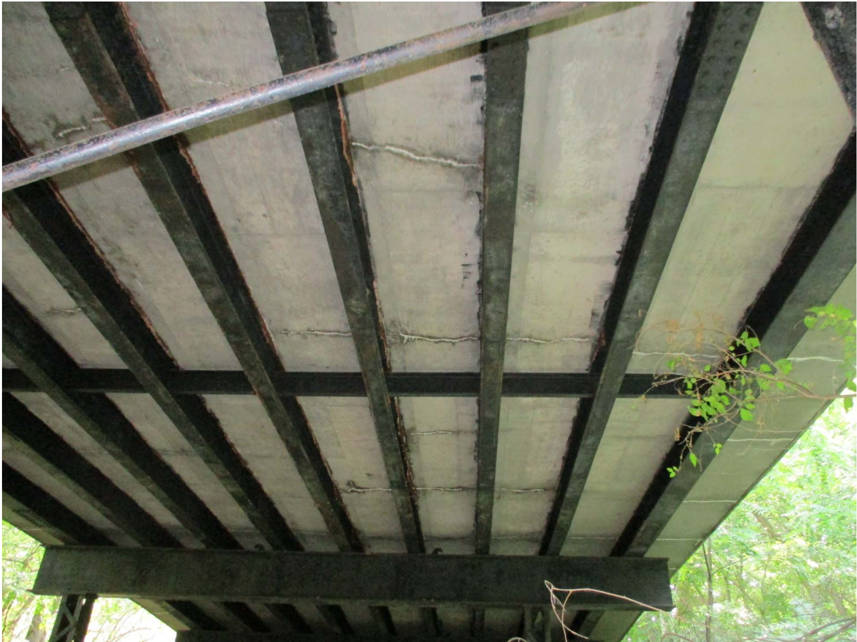
Center span deck bottom cracks
