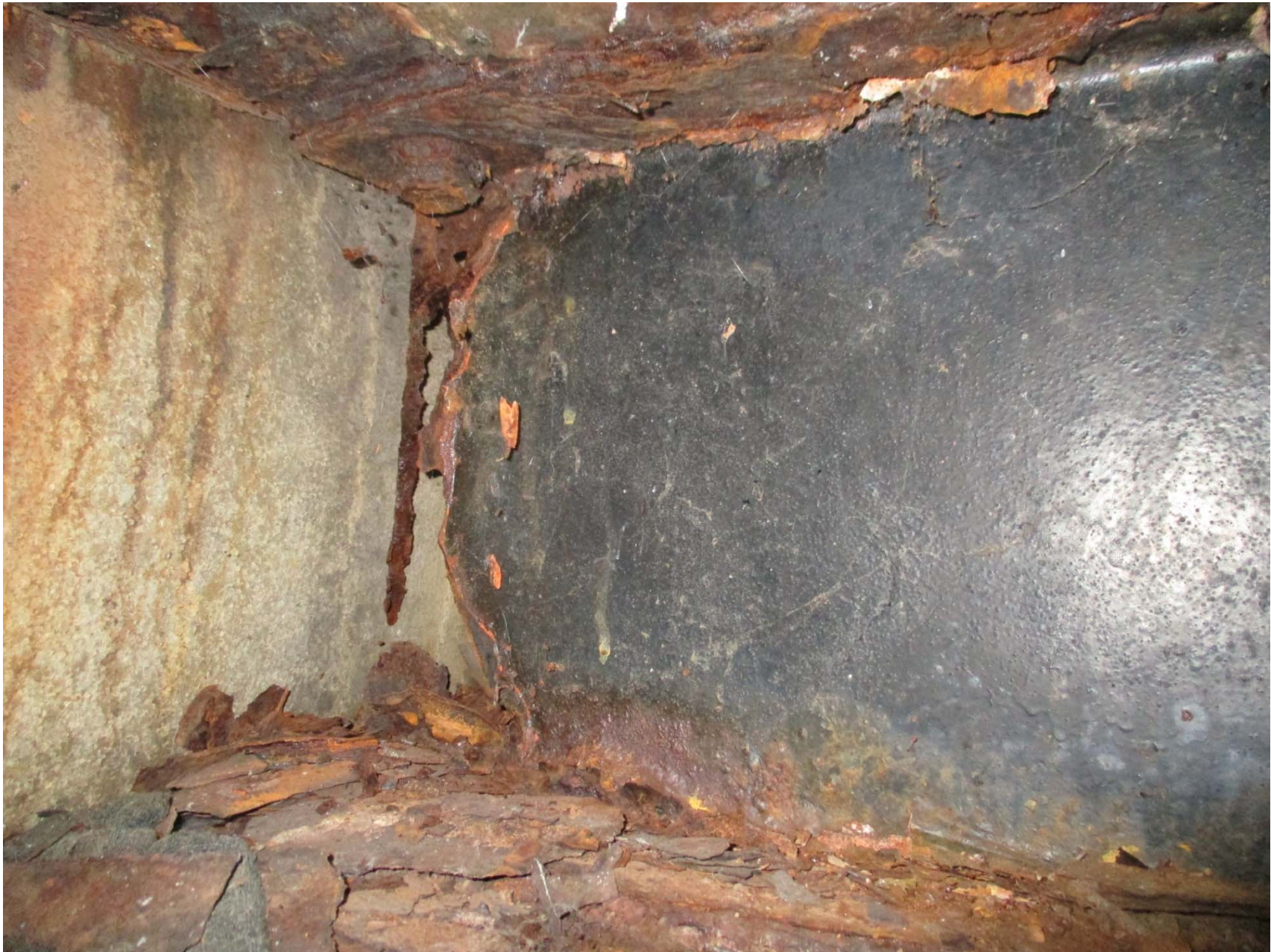
Beam 4S web mostly gone at the end, west abutment
