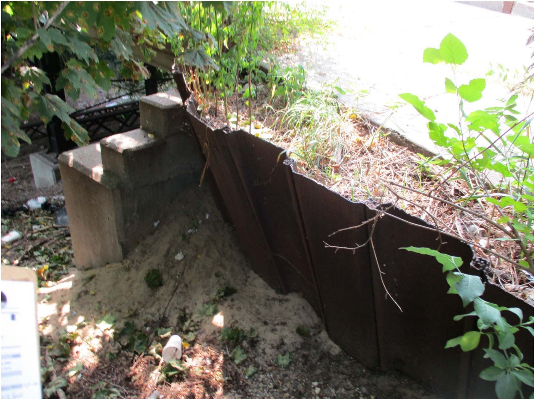
SE steel sheet wall failing, settlement and loss of fill at ends
