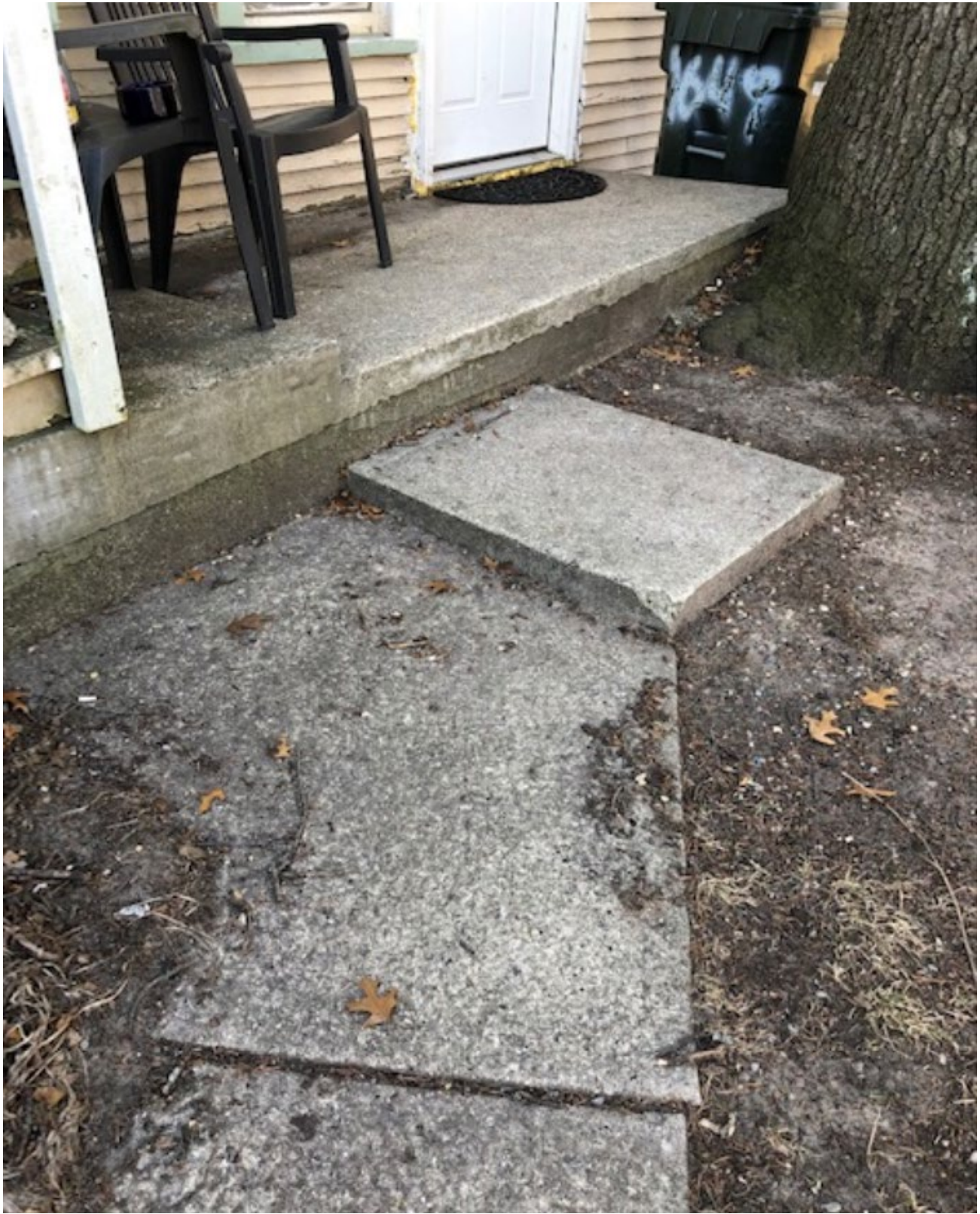
Existing cement porch is being pushed into the house by a growing tree
