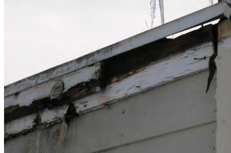
Hole in roofing/eave area.
