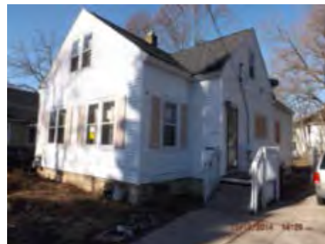
Side after fire-rear windows boarded.
