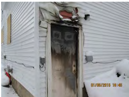
Rear of structure from fire.
