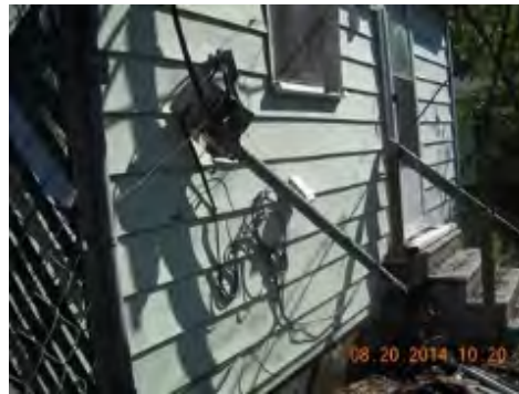
Electric mass knocked off of home.
