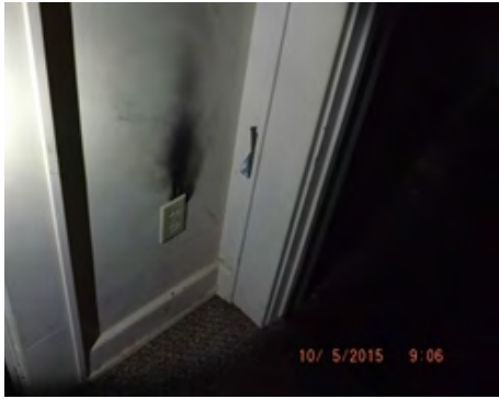
Interior electrical outlet.
