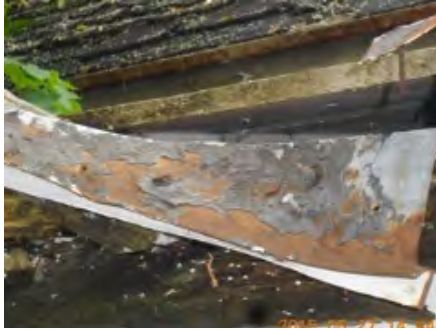
Roofing materials falling.
