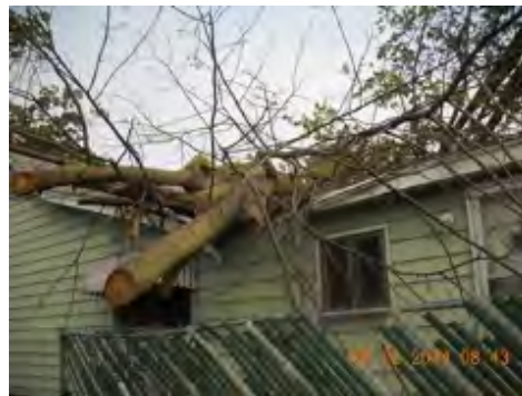
Tree on roof (south side).
