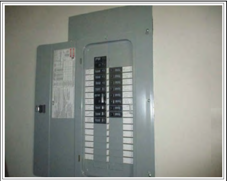
Electrical Box (Unit B - main level)
