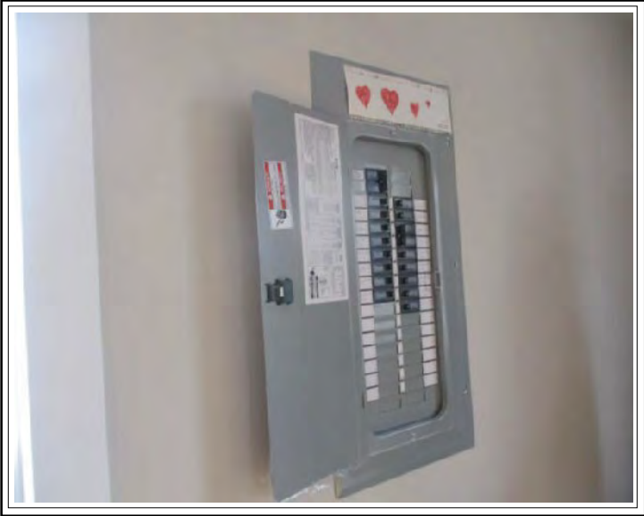
Electrical Box (Unit A - second level)
