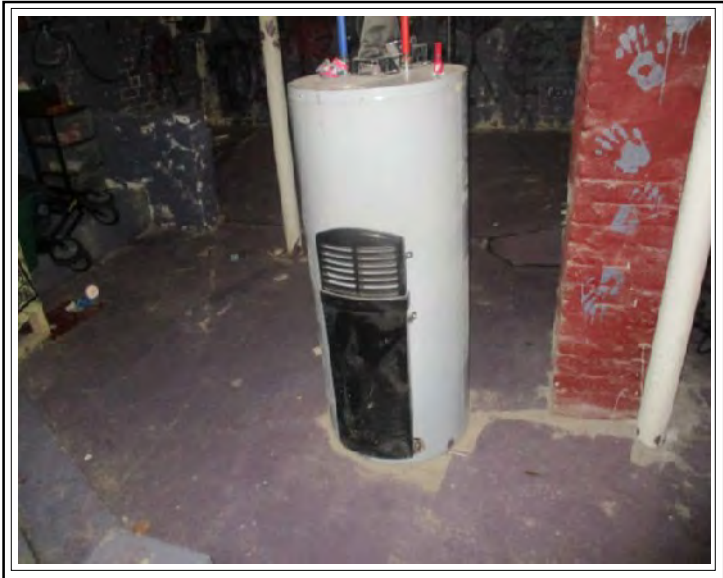
Water Heater (Unit B - basement)
