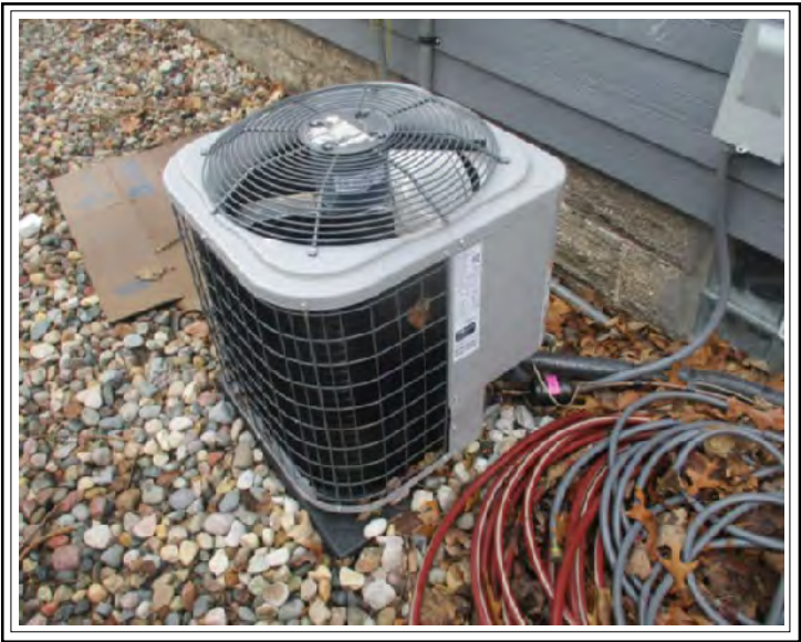
Central Air Unit
