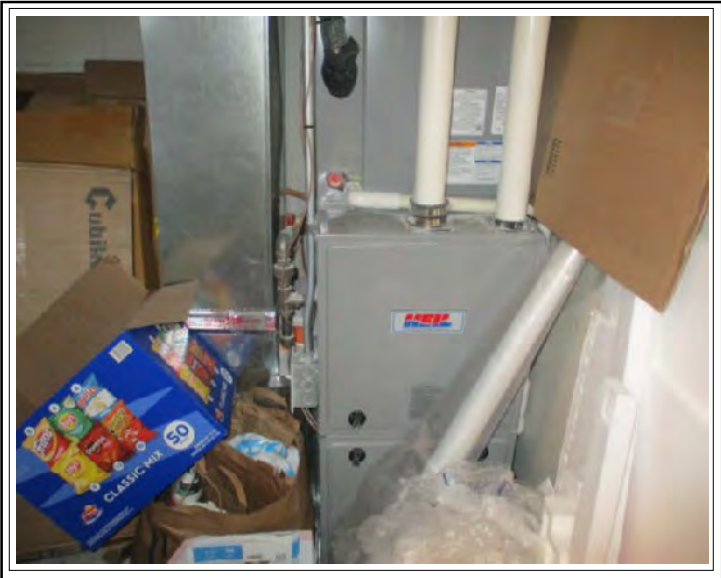
Furnace (Unit A - second level)
