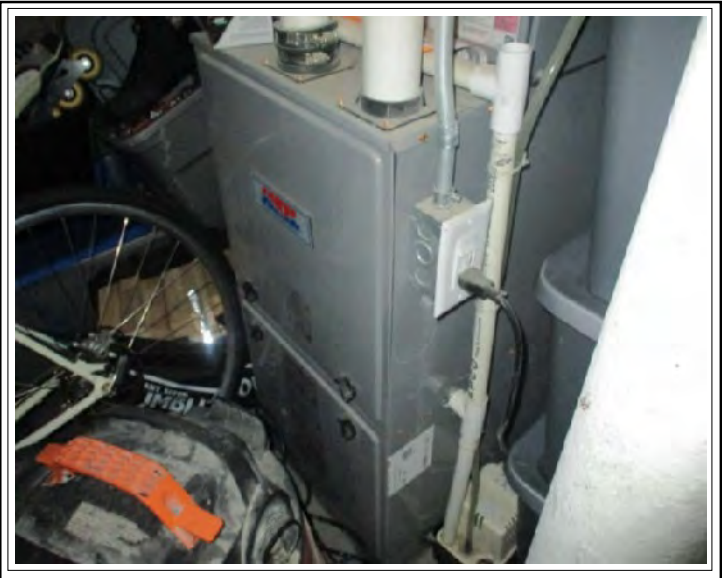
Furnace (Unit B - basement)
