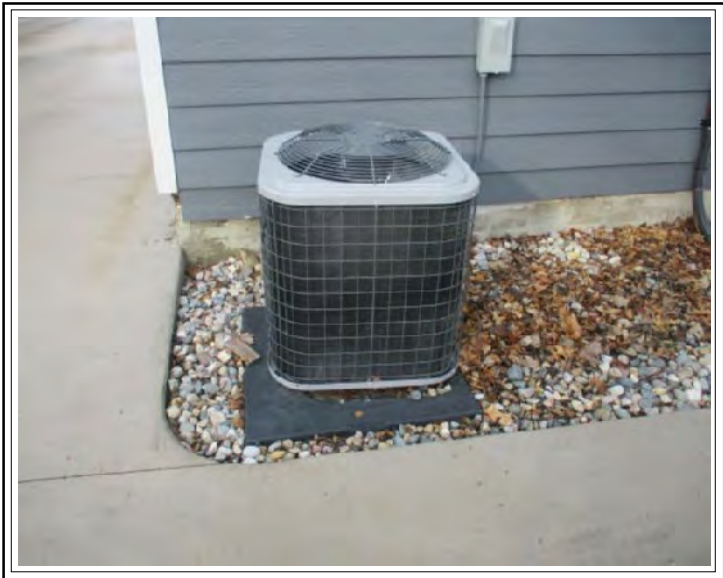
Central Air Unit
