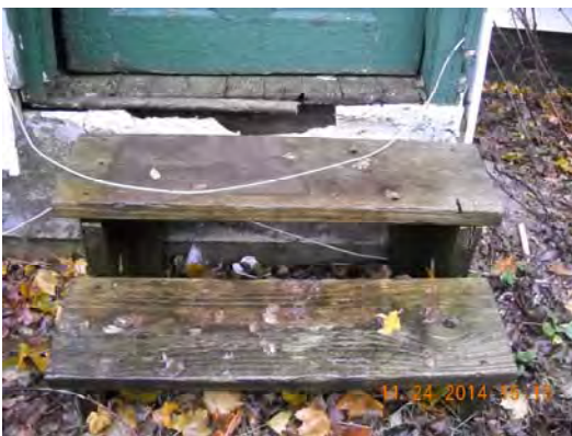
Rotted wood & foundation under door.
