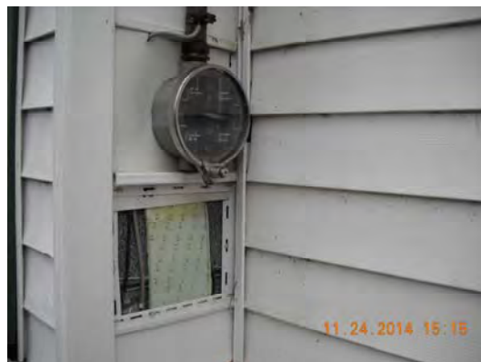
Electric meter gone & siding missing.
