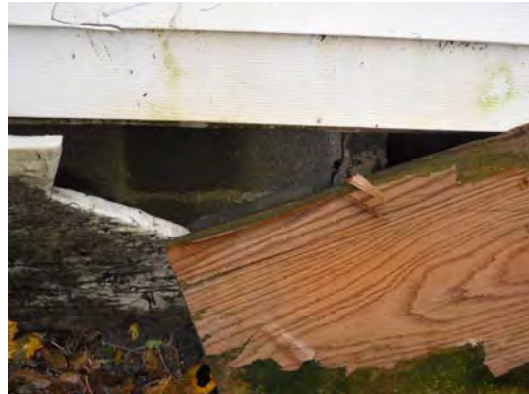
Hole in foundation.
