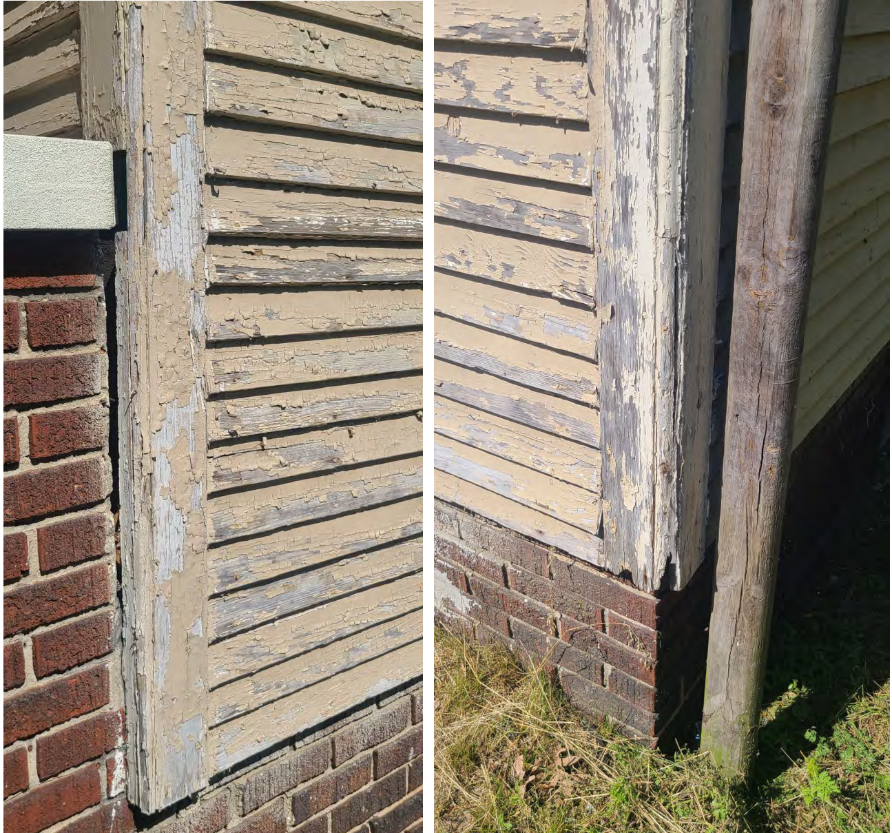
Photos depicting condition of existing wood siding proposed to be replaced with vinyl siding (#4)
