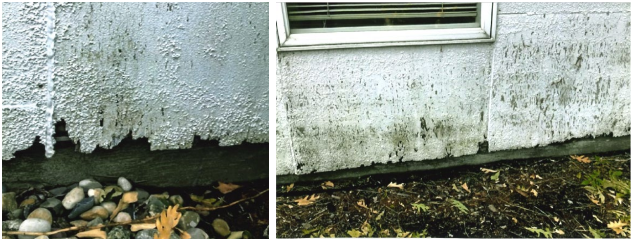
Detailed view of existing, deteriorated material.
