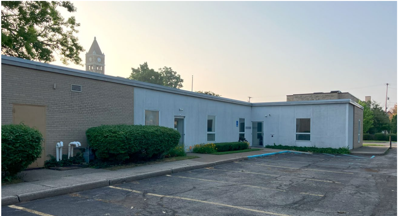
View of building from alley, looking east. All areas with white material are proposed to be replaced.
