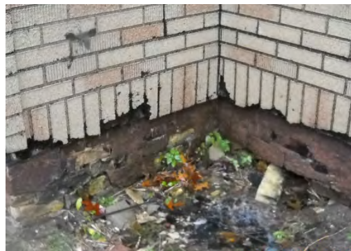
Foundation & siding deteriorating.
