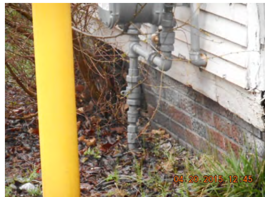
Foundation has bowing @ the gas meter.
