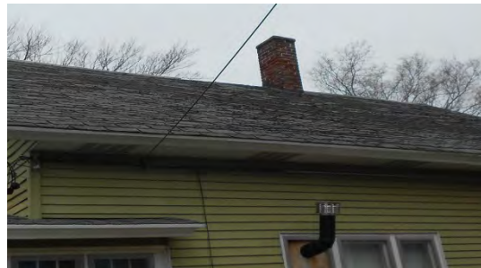
Deteriorated shingles on South side of home.
