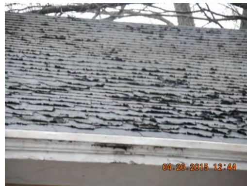
Shingles coming up/missing.
