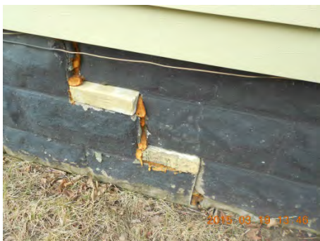
Foundation has some issues.
