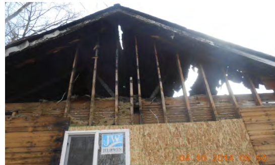
Rear of home-fire damaged.
