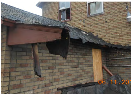
Rear roofing deteriorated.
