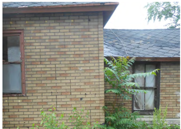
Roofing is deteriorated.
