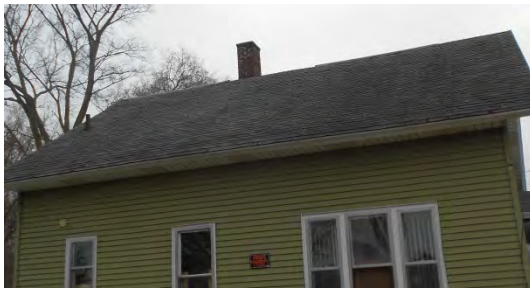
Some shingles are deteriorated on North side of home.
