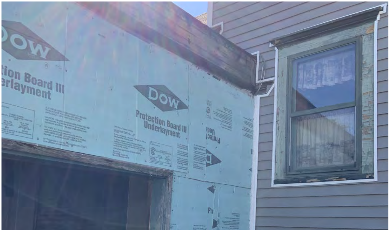
Connection to house on exterior of garage
