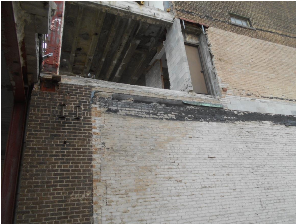
HA #35. Tar and Flashing on North Exterior wall of Older Section between 1 st and 2 nd Floors.
