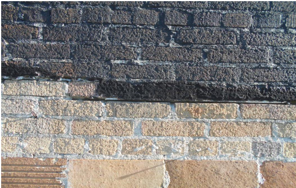
HA #5. Tar on Exterior of Rooftop Elevator/Mechanical Room.
