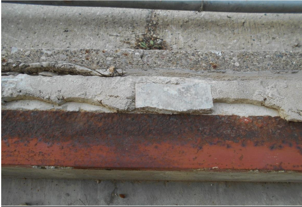
HA #29. Transite. Ground Floor of Older Building. Pieces stuck in Cement on Former Exterior Wall Foundations.
