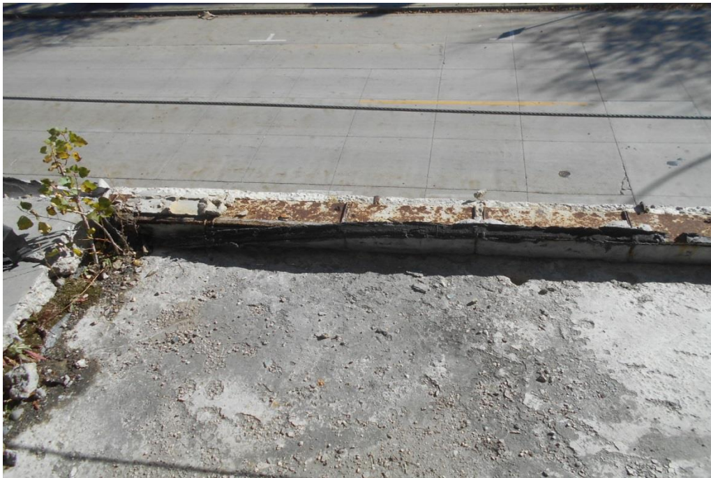
HA #22. Tar and Flashing at base of 2 nd floor South wall near Stairwell.
