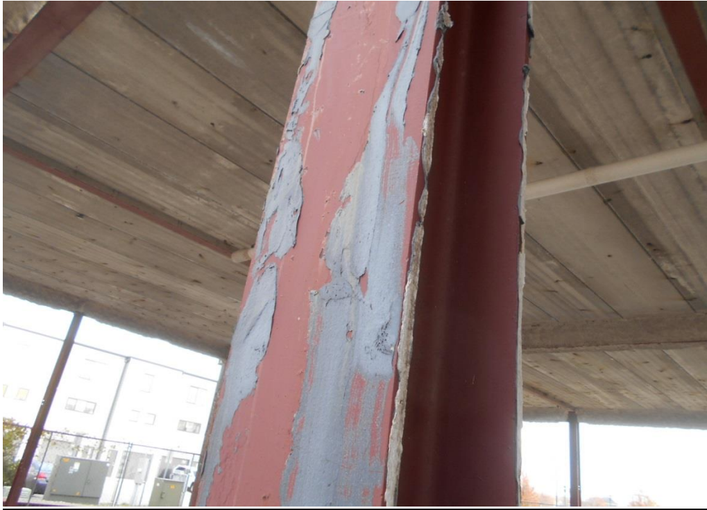
HA #34. Mastic on Steel Columns of Newer Addition.
