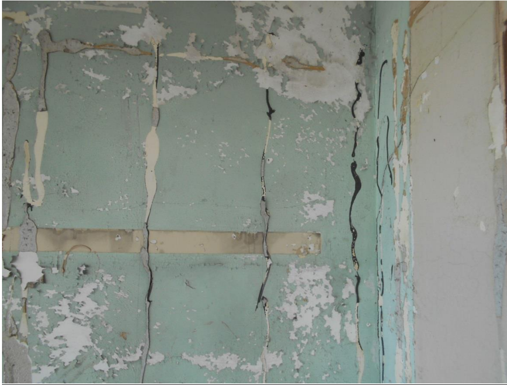
HA #12. Mastic on Plaster Walls (Behind Wallboard Systems)
