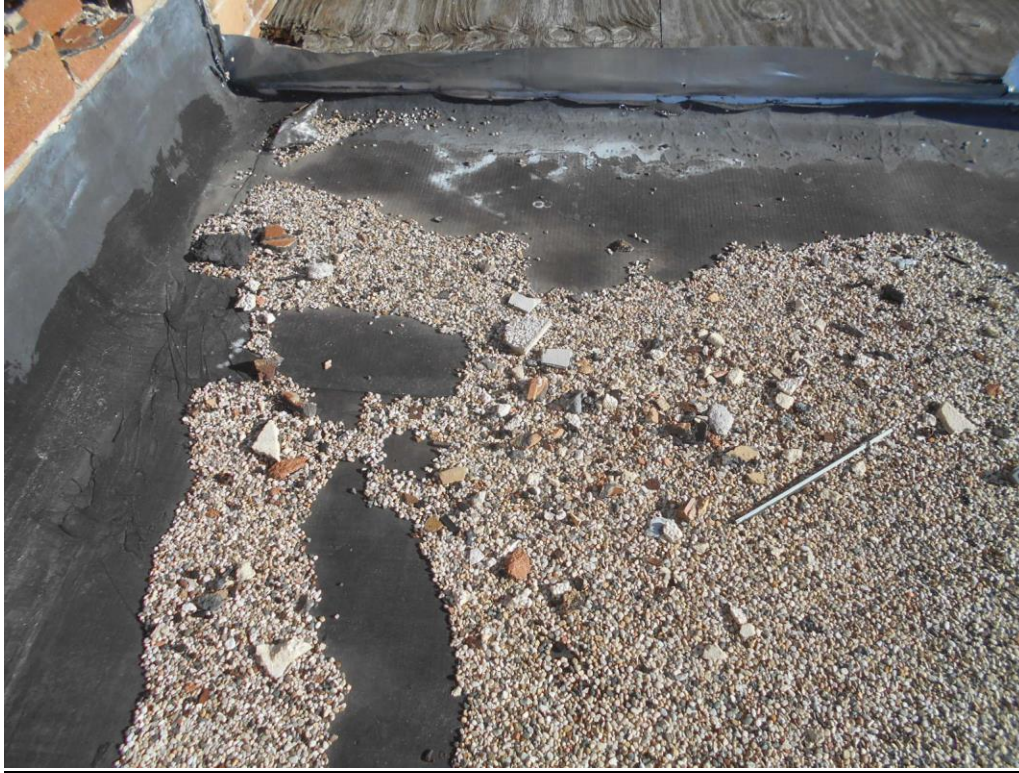
HA #6. Transite Debris on Older Building Roof.
