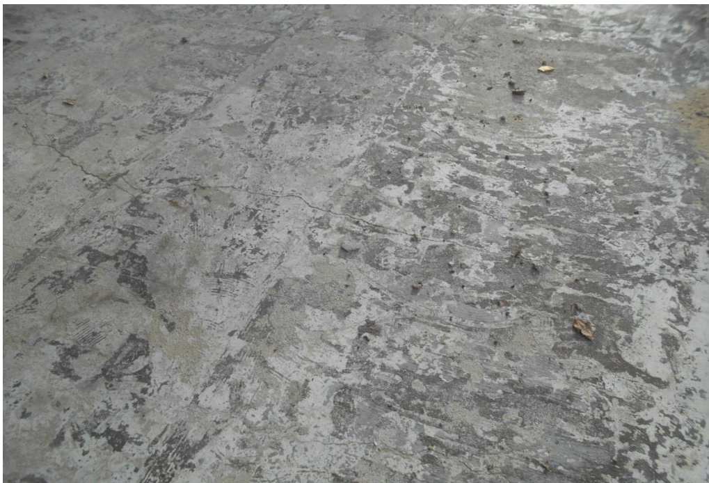
HA #32. Mastic, Black. Ground Floor Lobby.
