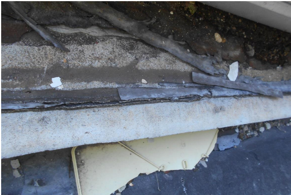
HA #24. Multiple Layers of Caulking/Sealants. 2 nd Floor/Newer Addition Roof.
