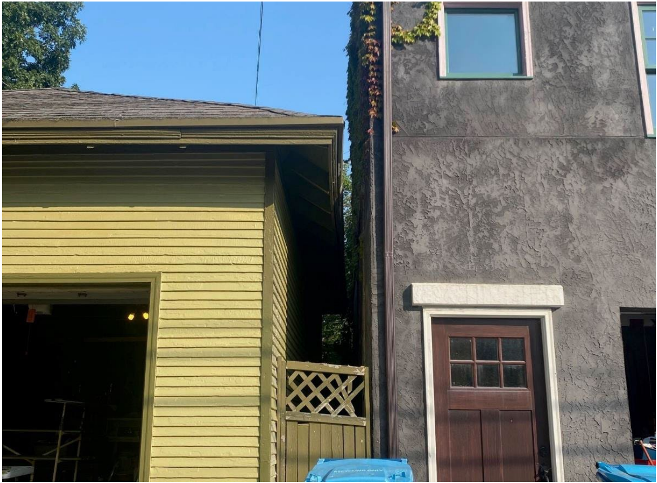
Northeast corner of the garage showing the tight clearance between the neighboring garage.
