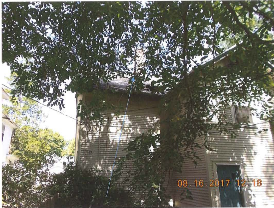
Large hole in roof from fire
