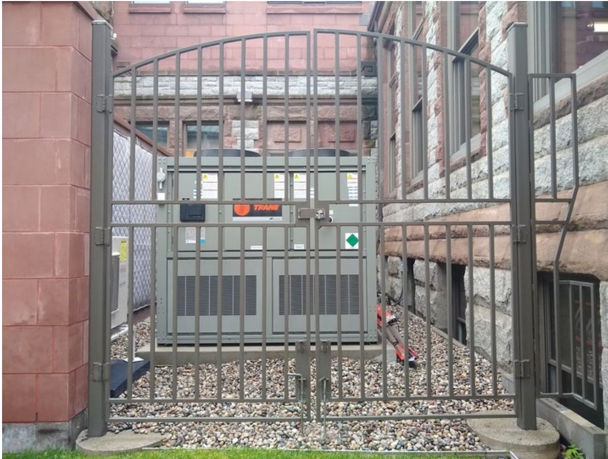
View of HVAC system space in courtyard and basement window wells.
