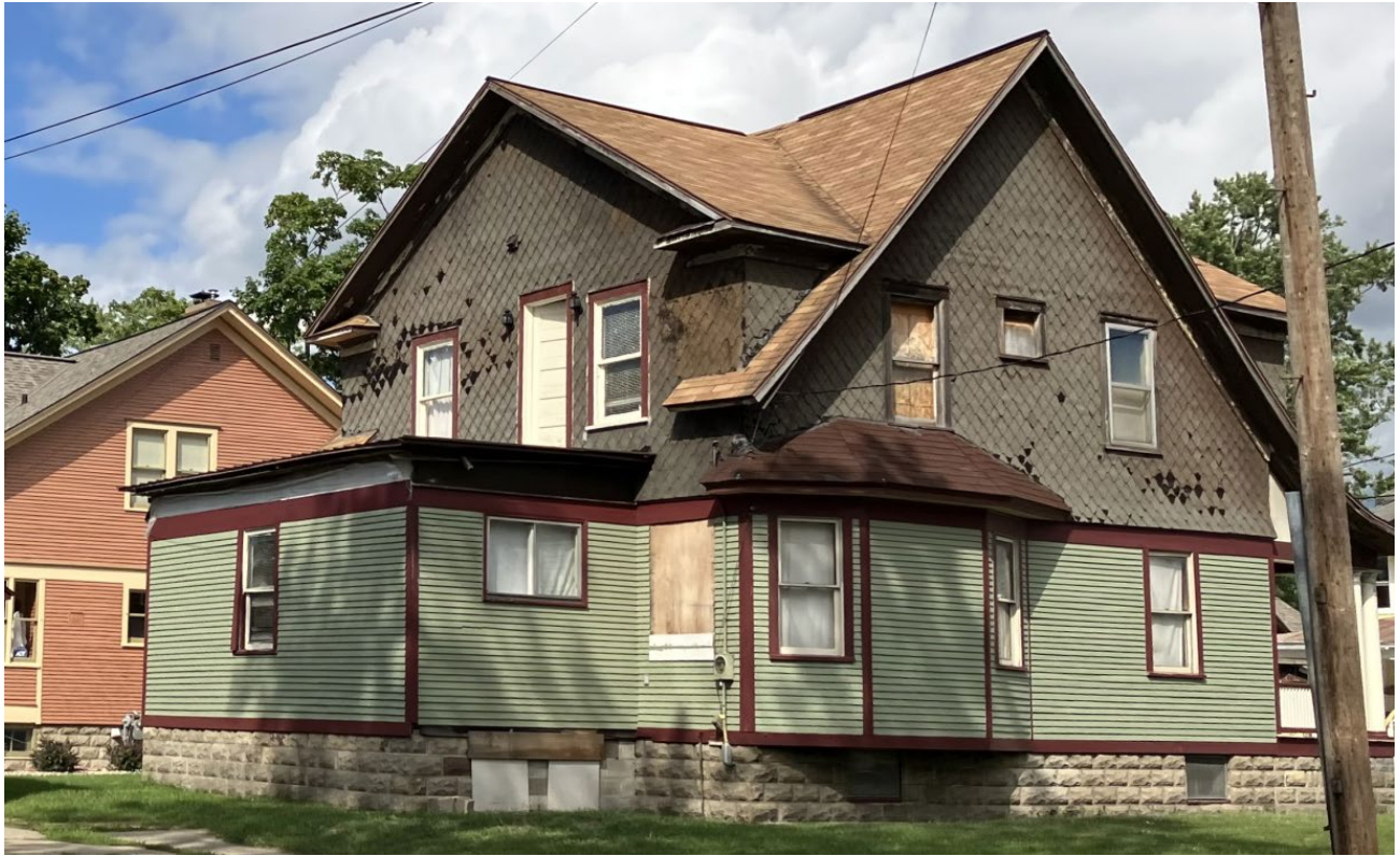
View of west (rear) and south elevations from E. Southern Avenue. Boarded-up first-story window is missing and proposed to be replaced. Two double-hung windows and one picture window on the second-story south elevation is proposed to be replaced.
