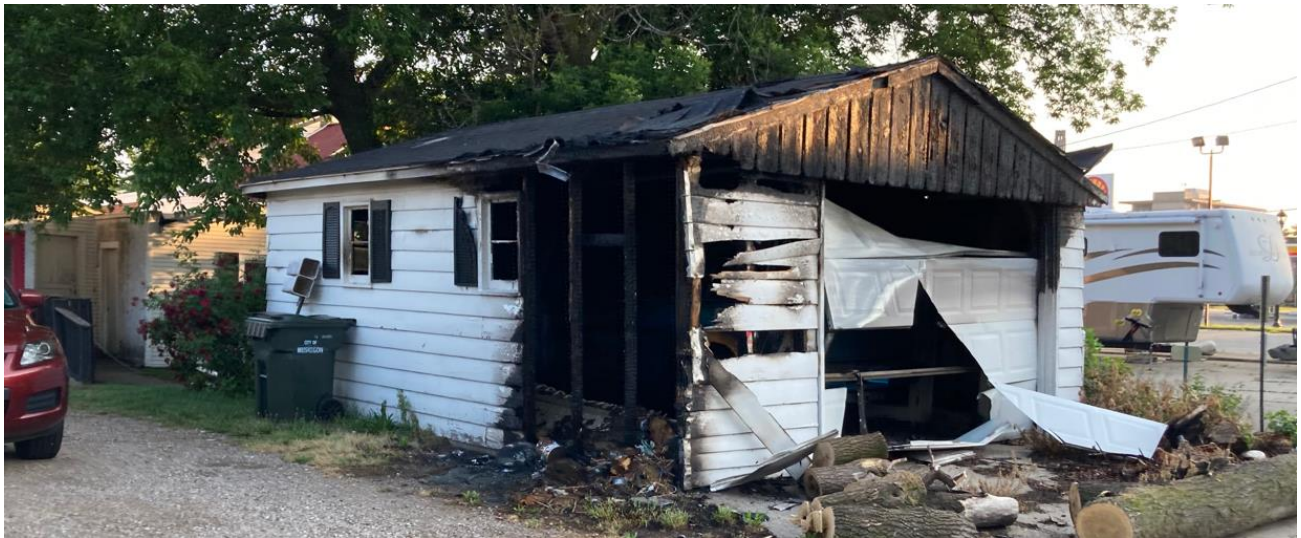
View of fire damaged, detached garage looking north from alley (June 2021)
