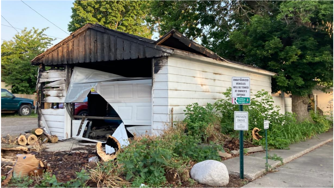
View of detached garage looking west from alley after fire (June 2021)
