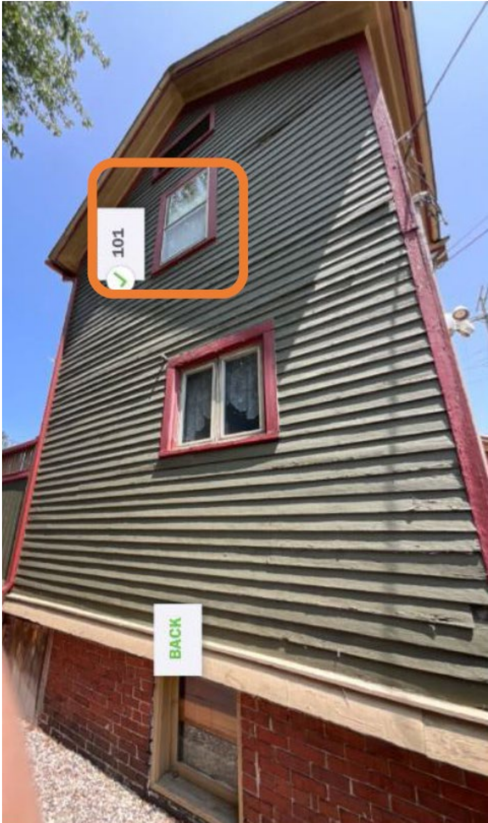
One second-story window on the west elevation proposed to be replaced.
