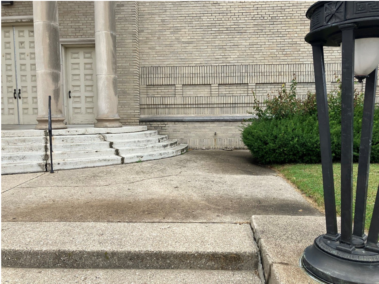
View of the proposed ramp location where it will rise from the plaza level to the top of the entrance steps.
