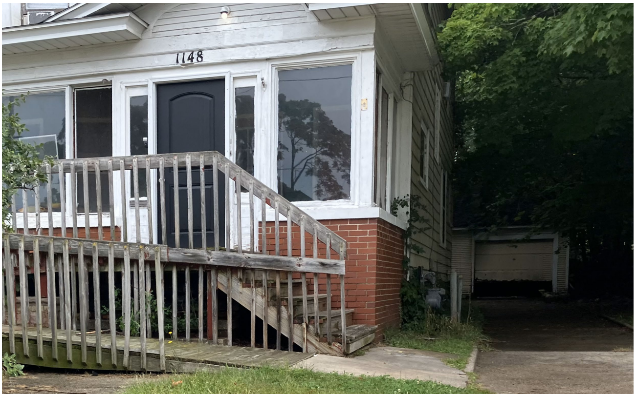
Detail view of front porch with section of original wood siding visible above front door.
