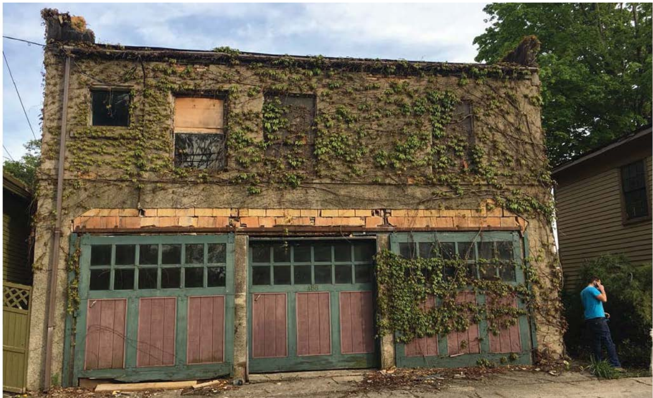
Current condition of rear wall, exposed clay masonry blocks where former awning attached
