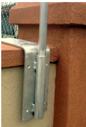
Bracket supporting parapet mounted pole
