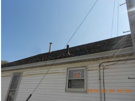
West side bad roof.
