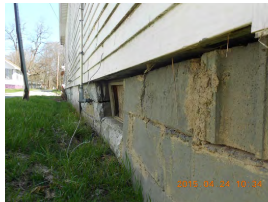
West side foundation buckling.
