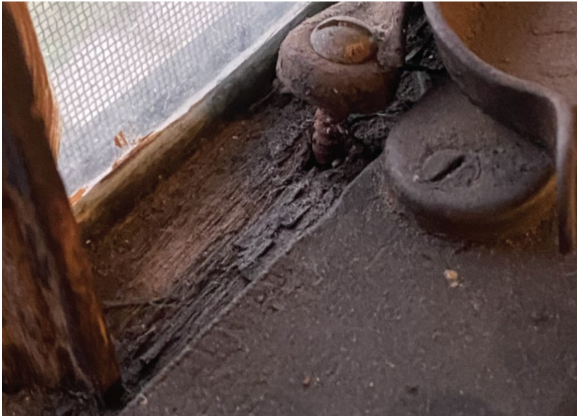
Interior deterioration of windows.
