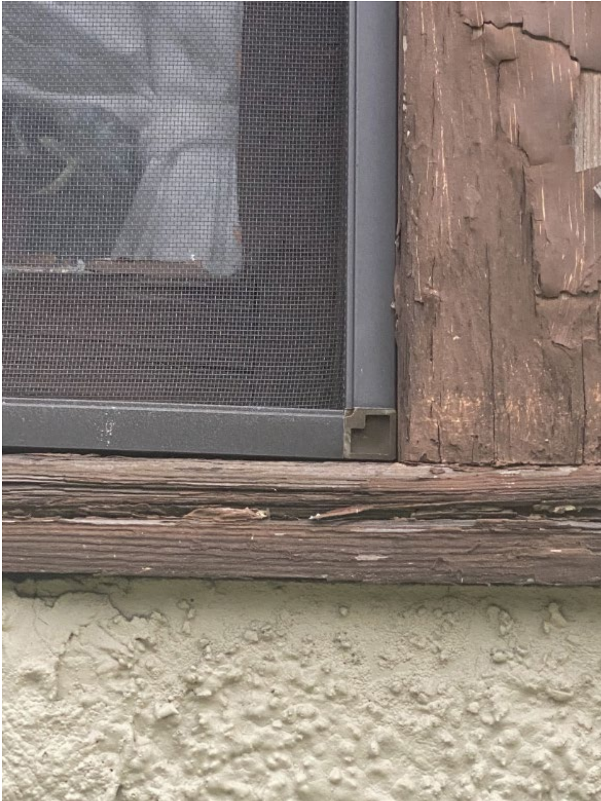
Exterior deterioration of window frames.
