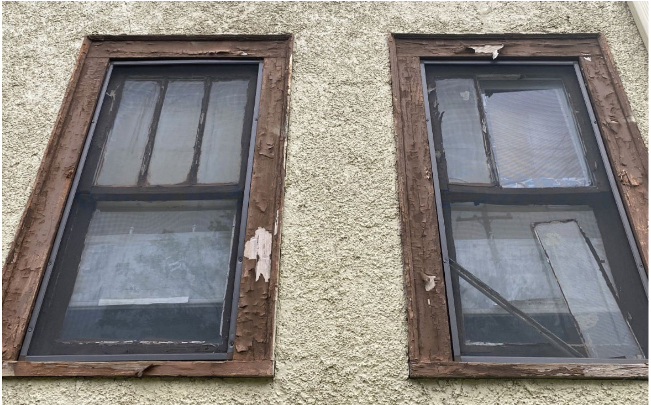
Exterior deterioration of windows and window frames.
