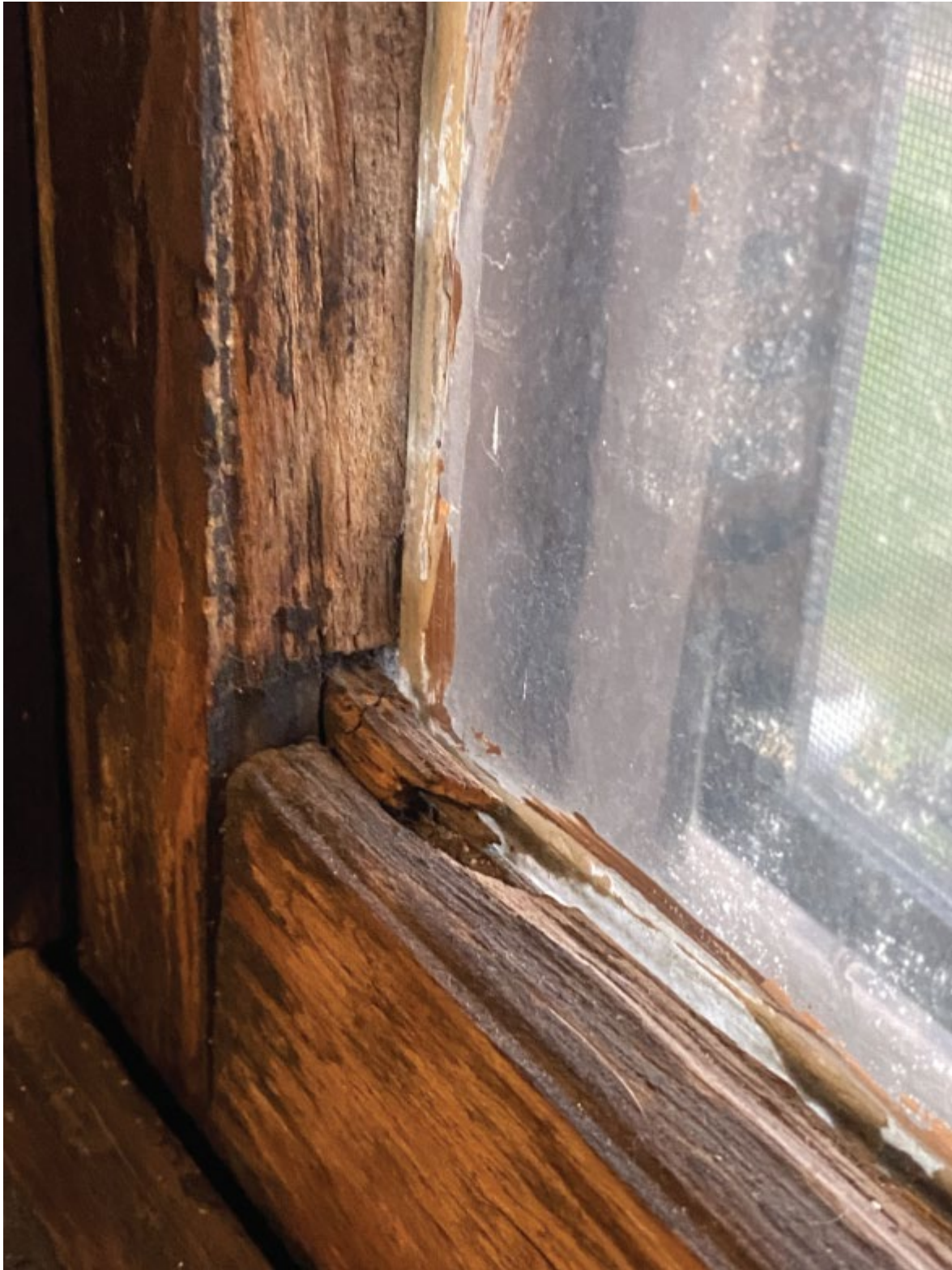
Interior deterioration of windows.
