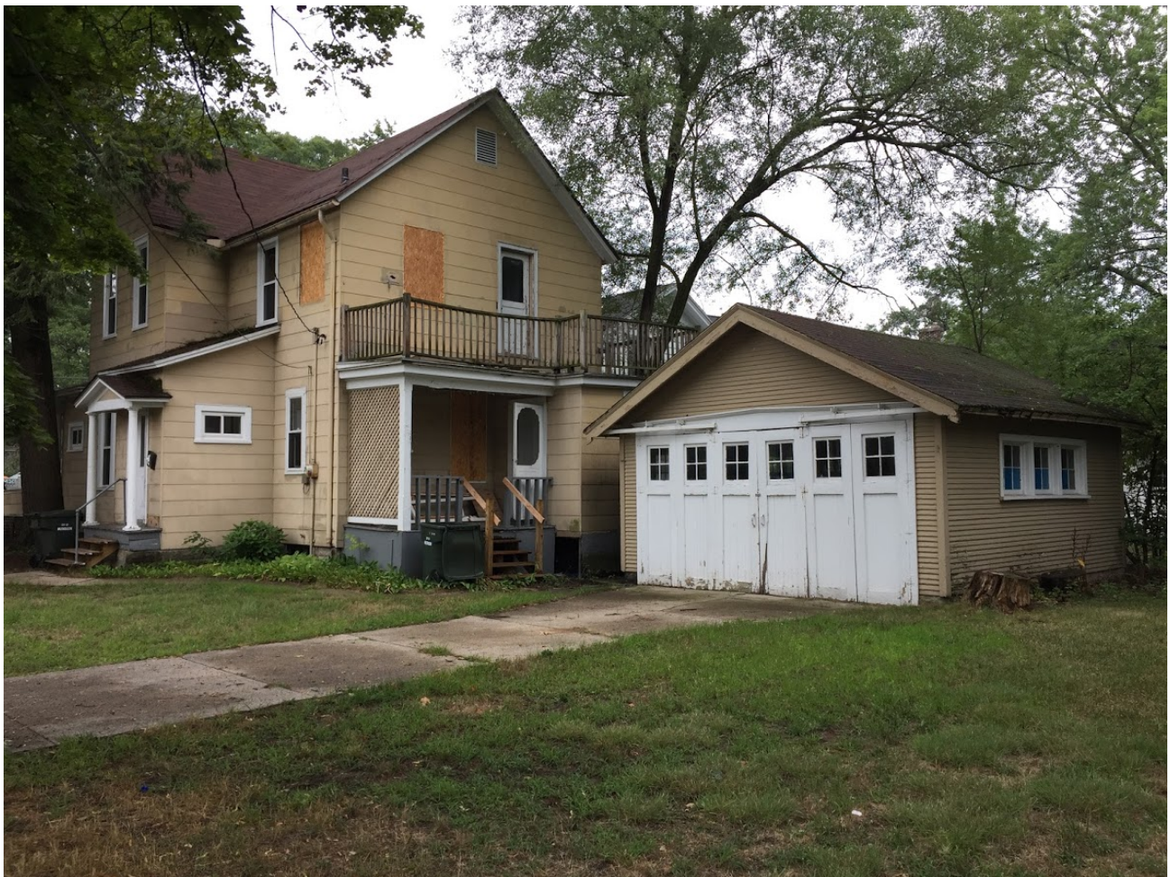
2018 photo showing boarded-up windows on North and West façades of 1561 Peck (viewed from Southern Ave.)
