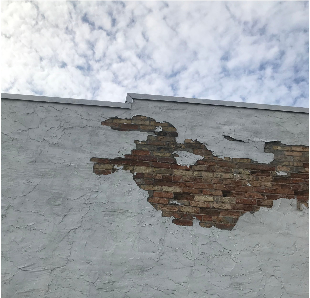
View of damaged area, exposing brick. Wall was sealed a few years ago, but damage continues
