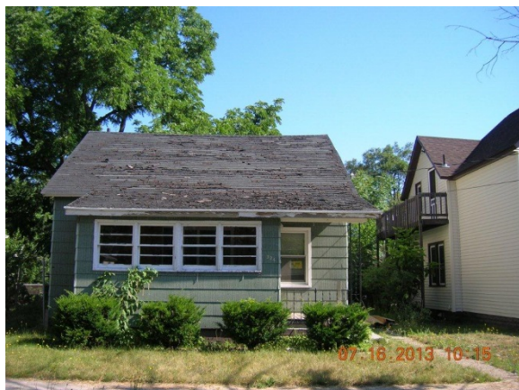
224 W Grand photos taken by Code Compliance Inspector
