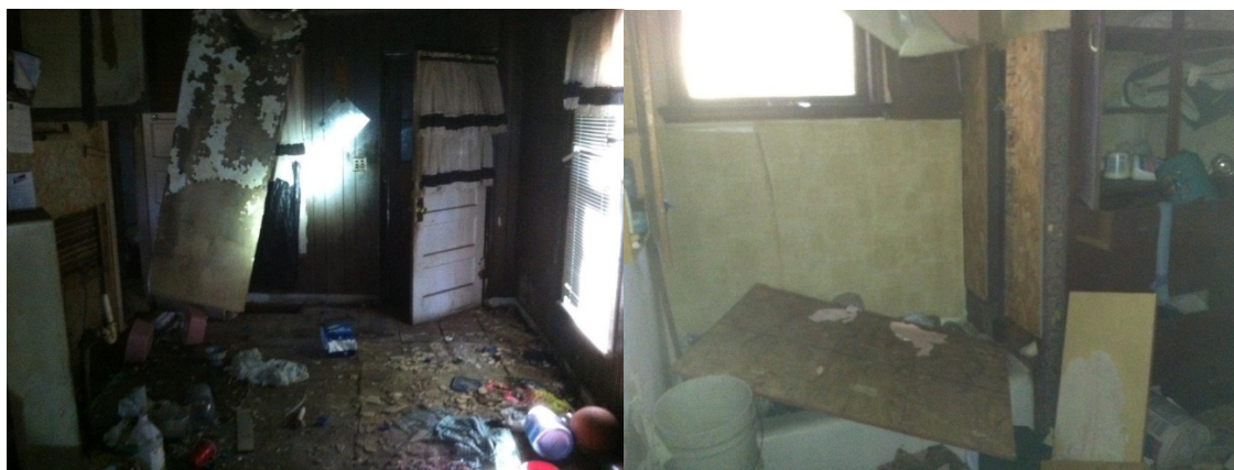
1324 Pine – Pictures provided by Code Compliance Inspector, Board up Contractor &SAFEbuilt
