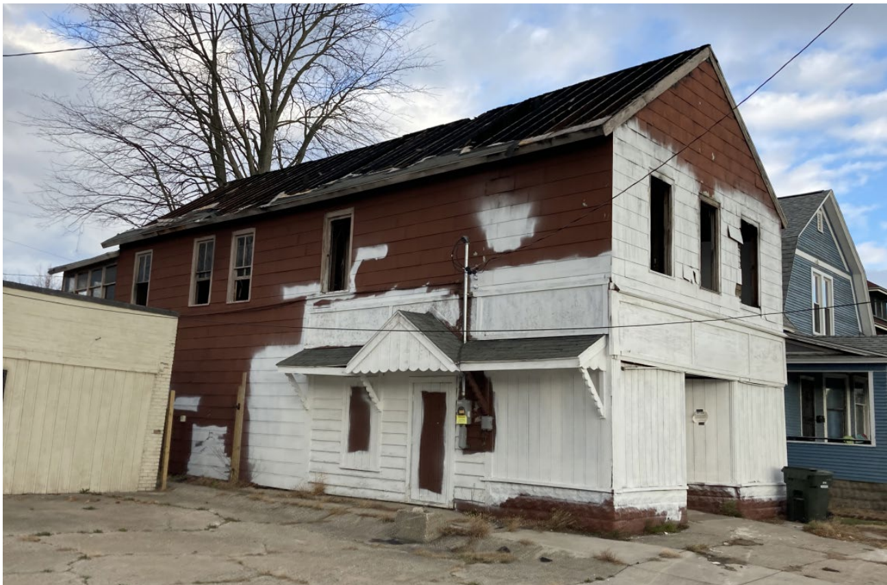
A similar view today, with fire damage visible on second floor
