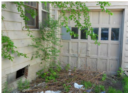
Foundation by garage buckling.
