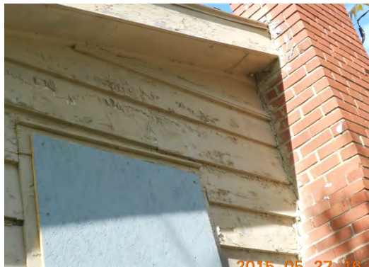
Chimney mortar deteriorated in spots.
